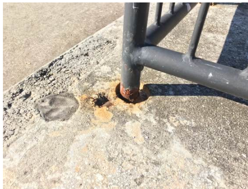
Repaint Parking Deck Handrail. Caulk Post Pockets To Prevent Holding Water And Rust
