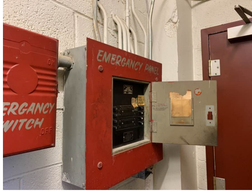
Existing Emergency Panel In Storage 17 Needs To Be Replaced
