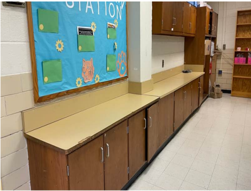
Cabinetry Is Beyond Useful Life And Needs To Be Replaced
