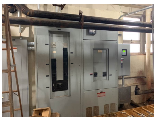
Main Switchboard In Mechanical Room 36.1 Is Beyond Its Useful Life. Photo Should Be In Building 2012
