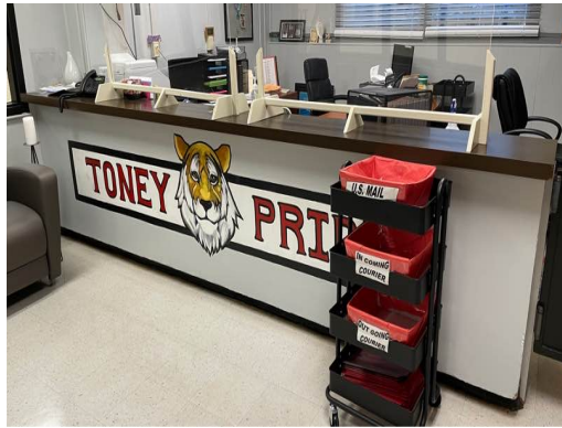
Main Office Counter It Is Non-ADA Compliant. Counter Needs To Be Retrofitted To Provide ADA Accessibility
