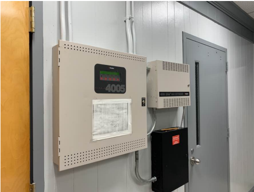
Existing Fire Alarm System Is Beyond Useful Life
