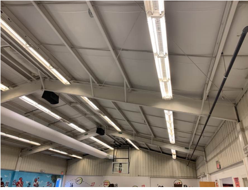
Existing T8 Fluorescent Lamps Are Beyond Useful Life
