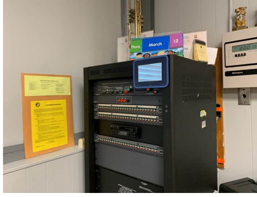
The Existing Intercom System Is Beyond Useful Life
