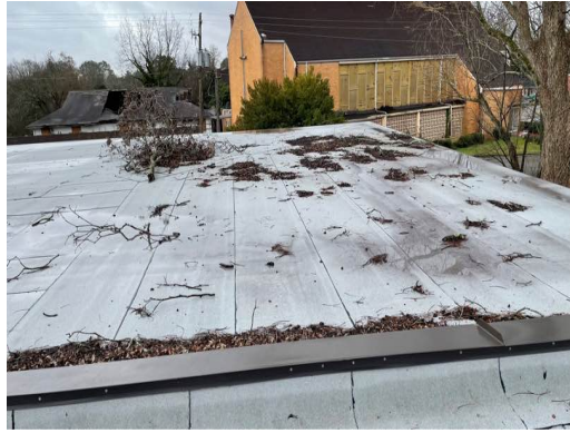
Roof Debris Needs To Be Cleared
