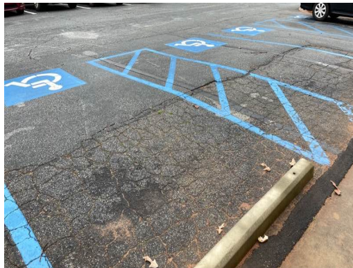
Asphalt Parking Area Is Cracked And Beyond Useful Life Needs To Be Repaved
