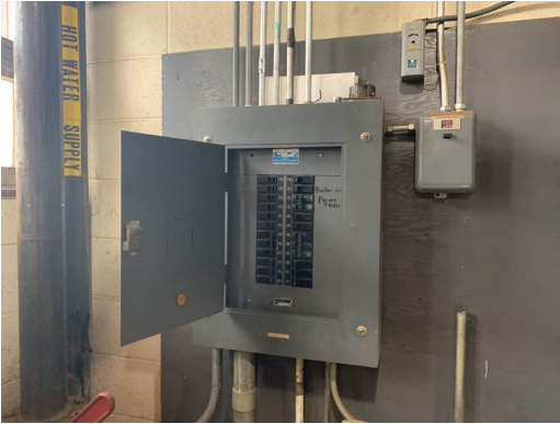
Electrical Panel In Mechanical Room 36.1 Is Beyond Its Useful Life. Photo Should Be In Building 2012
