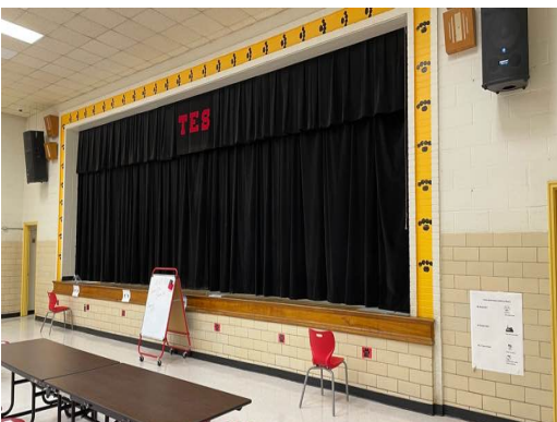
Stage Access Is Non-ADA Compliant And A Lift Is Needed To Provide ADA Accessibility
