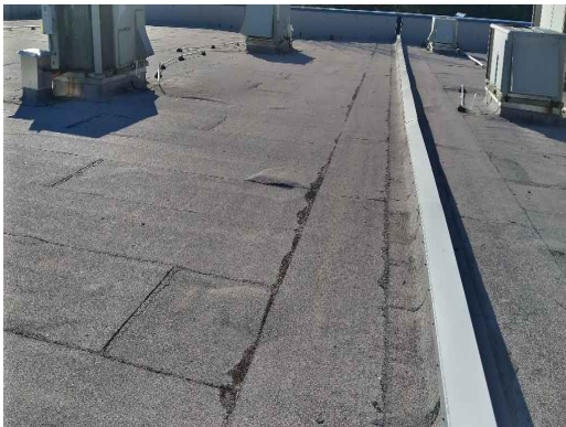
Roof Major Blisters
