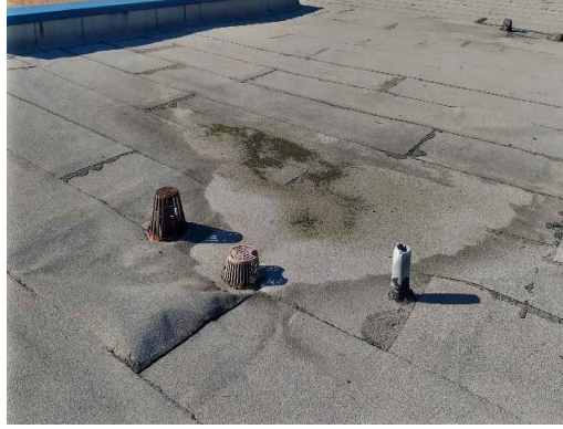
Roof Deficiency Conditions
