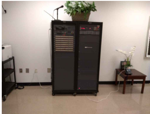
Security System Is 20 Years Old
