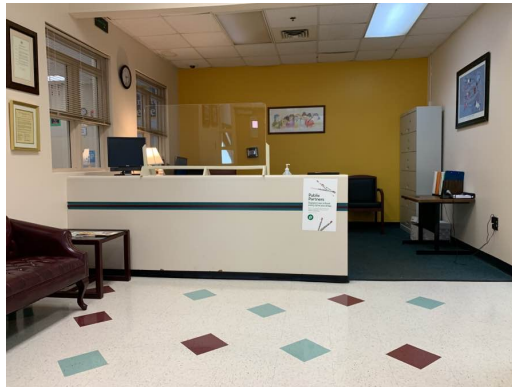
Counter Does Not Meet ADA Requirements
