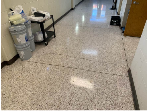
Cracked Terrazzo In Corridor
