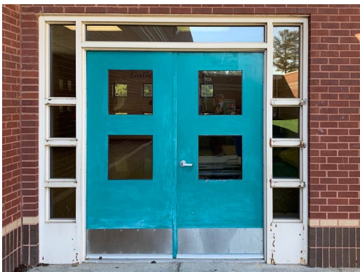
Exterior Storefront Frames Are Rusted
