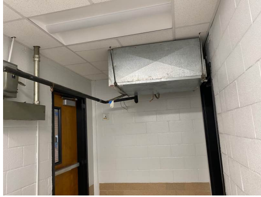
2010-2011-2012- Water Source Heat Pumps And Exterior Wood Door - Replace All - Entire Building
