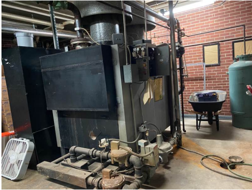
2010- Mech-204.1- Boiler - Replace
