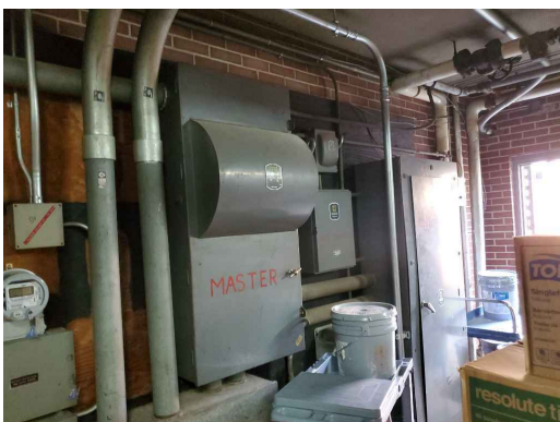
600 Amp Main Disconnect Beyond Useful Life
