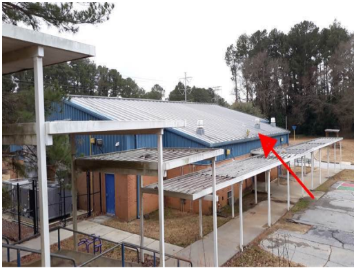
Roof Gutters With Debris And Tree Growing Need To Be Cleaned
