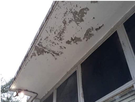
Concrete Roof Overhangs With Peeling Paint Need To Be Repainted
