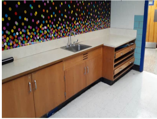
Classroom Wood Cabinetry Beyond Useful Life Needs Replacement
