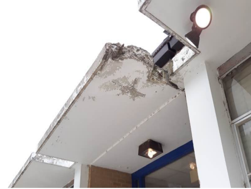
Concrete Roof Overhangs Water Damaged And Falling Apart And Need To Be Repaired. Structural Study Recommended To Assess Concrete Structure Condition
