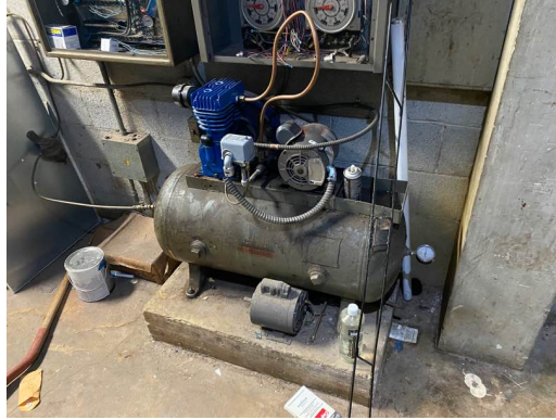
Existing Compressor Can Be Removed When Controls Are Replaced
