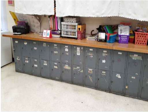
Classroom Lockers Beyond Useful Life Need Replacement
