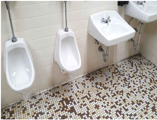
Restroom Tile Needs Replacement
