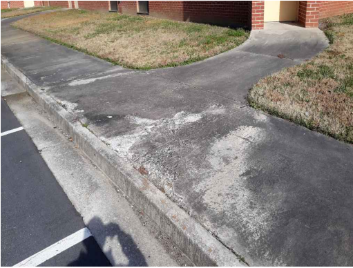
Site Spalling Concrete Sidewalks Need Replacement
