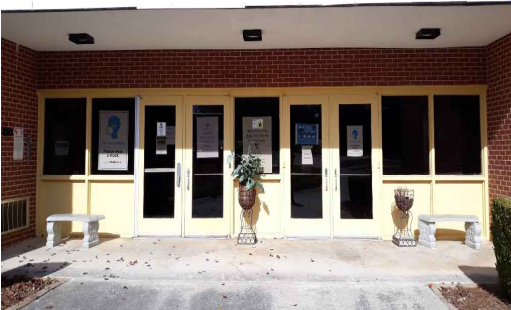
Main Entrance Storefront System Beyond Useful Life Needs Replacement
