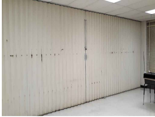
Folding Wall Partitions Beyond Useful Life Needs Replacement
