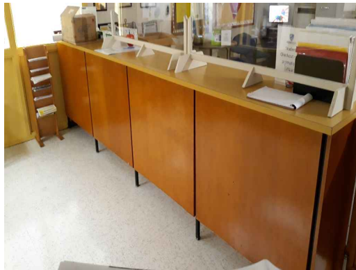
Main Office Welcome Counter Needs To Be Adapted For ADA
