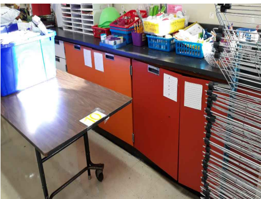
Cabinetry At Art Classroom Beyond Useful Life Needs Replacement
