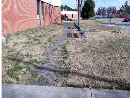
Crumbling Asphalt Sidewalks Need Replacement
