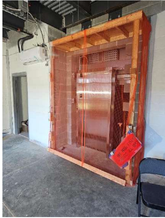
New elevator installed.
