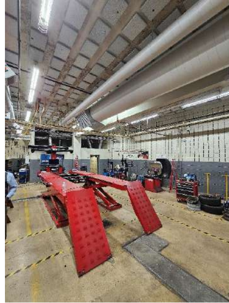
HVAC Duct to be adjusted in the Auto Lab.
