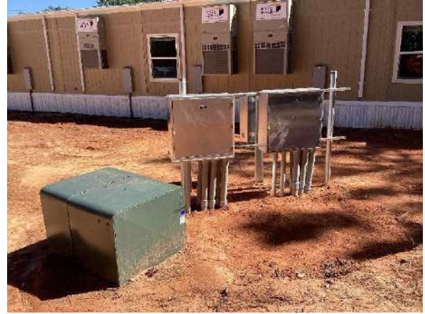
New transformer near modular buildings.
