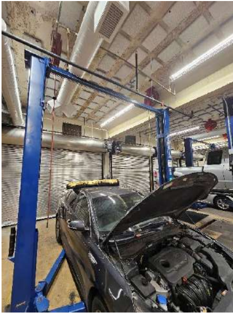
Fire Sprinkler lines to be adjusted in the Auto Lab.
