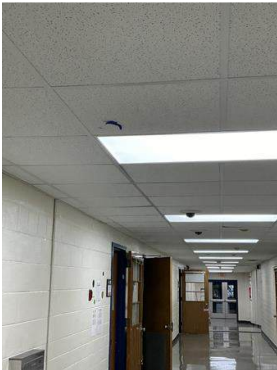
New ceiling grid and ceiling tile installed throughout the building. The floors are stripped and waxed.
