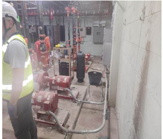
Piping for the new Chiller and new equipment Mechanical Room.
