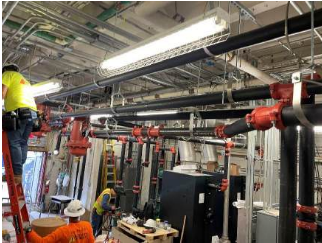
New equipment in the boiler room.
