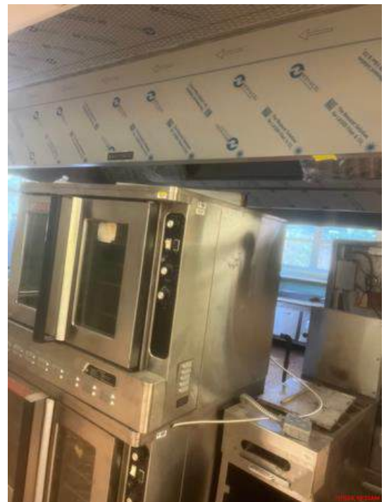
New kitchen hood installed
