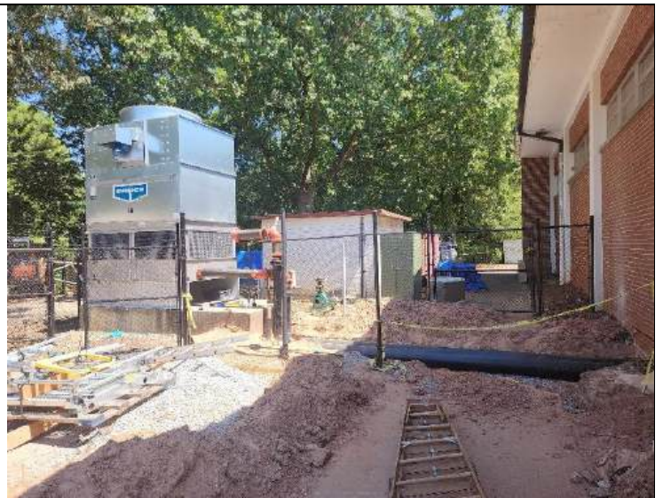
New Cooling Tower
