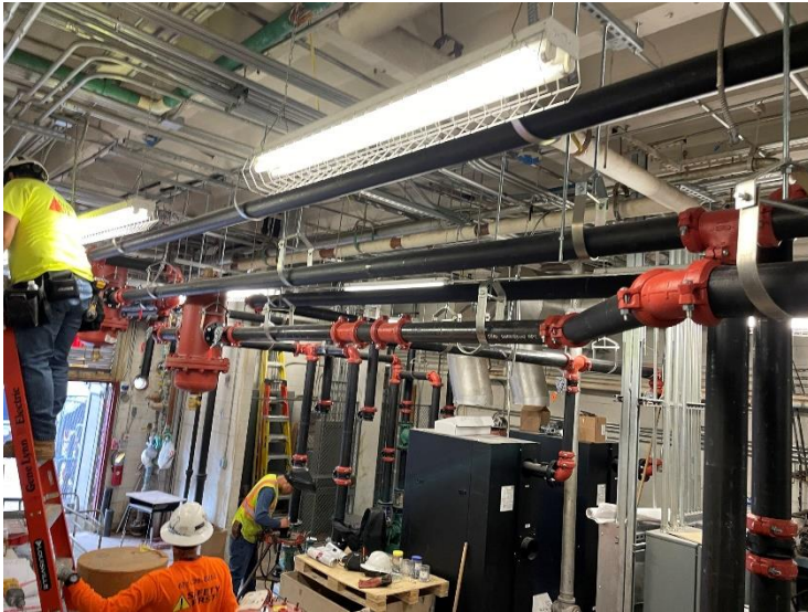
New equipment in the boiler room.
