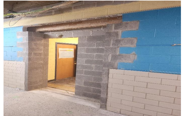
Demolition and Rebuild the two Doors into the Media Center for Emergency Egress
