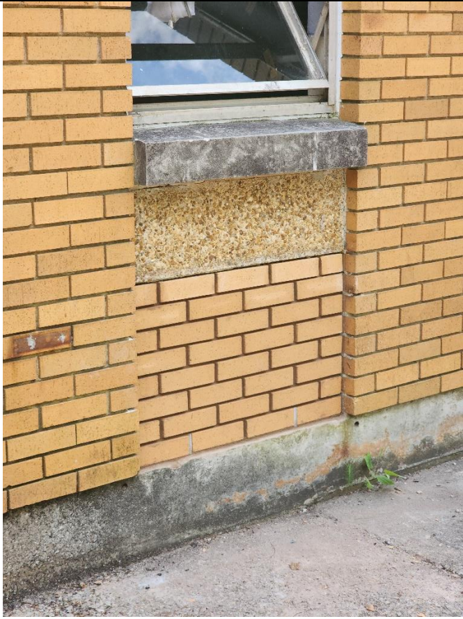
Exterior Wall Panel Repairs of the Opening left by the removal of the old units.
