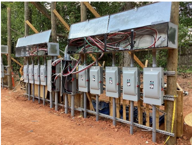
Electrical panels for the modular buildings.
