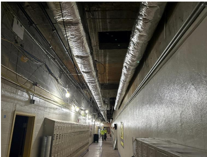
Fire Sprinklers and Insulated HVAC ducts in the corridors.
