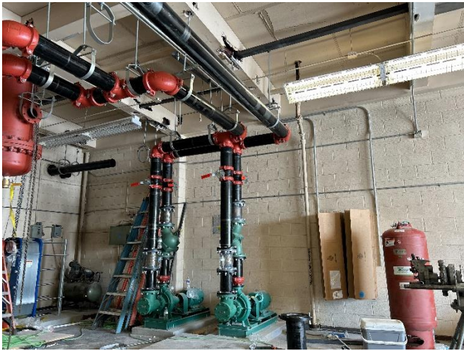
New equipment at the Boiler Room.
