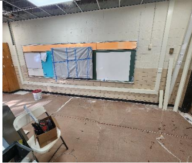
Mock up of Electrical Raceway
