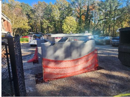
Supports for Cooling Tower
