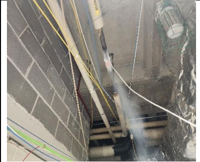
Freezing Existing Pipe to cut off to seal area for asbestos abatement and Demo
