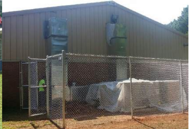
Gym RTU units
