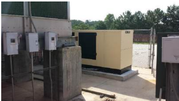
New generator at Freedom MS
