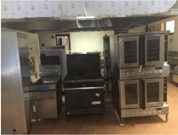
New Kitchen Equipment
