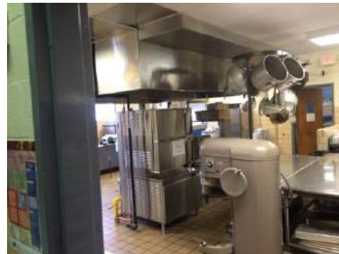
New kitchen equipment installed
