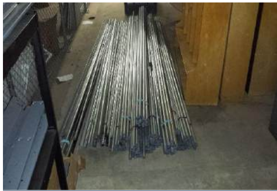
Conduit piping at Jolly ES
