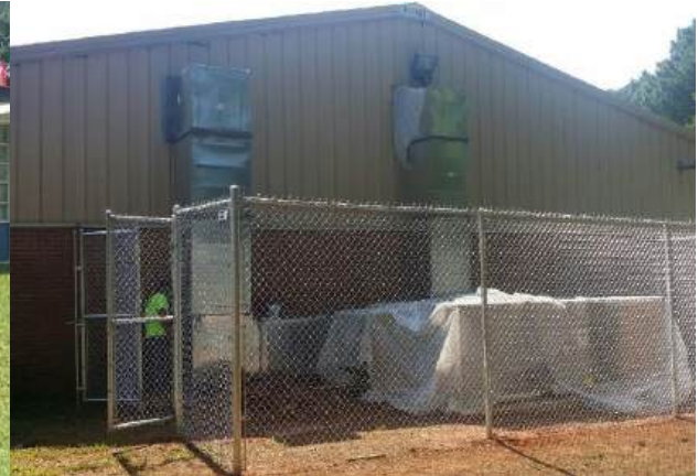
Gym RTU units
