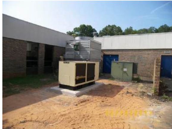
New Emergency Generator has been installed
