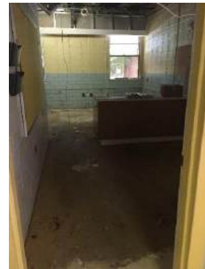
Classroom Lighting to be Replaced
