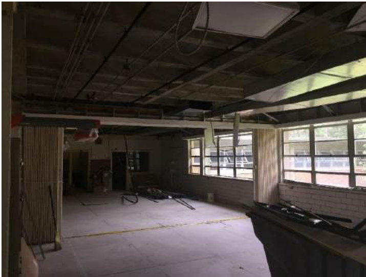
Cafeteria Lighting to be Replaced
