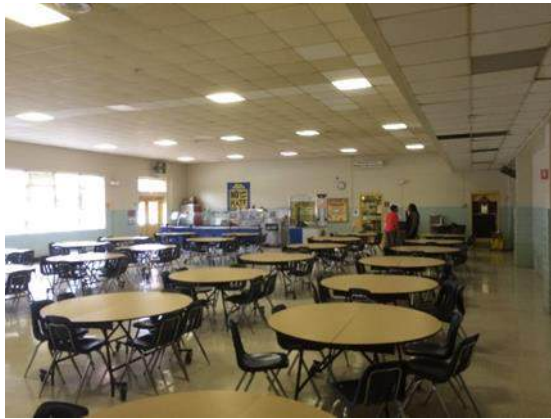
Cafeteria Lighting to be Replaced
