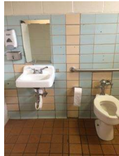
Bathroom fixtures to be replaced
