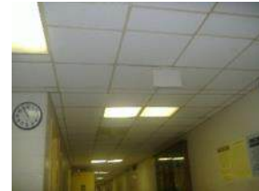
Hall Lighting to be Replaced
