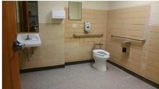
Chapel Hill ES Restroom after Construction
