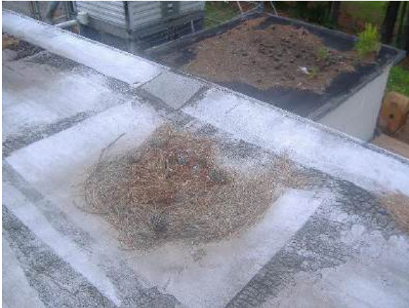
View of the roof drain clogged with debris
