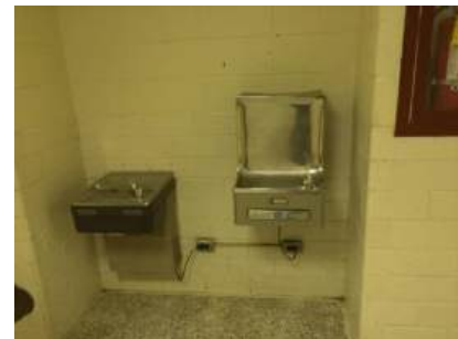
Water fountain fixtures to be replaced
