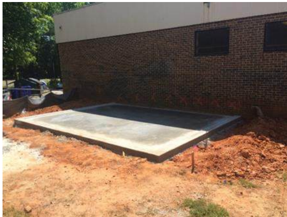
New cooler/ Freezer concrete pad has been poured and preparations are being made for the installation of a new Cooler / Freezer.
