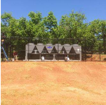
New Chiller Installed
