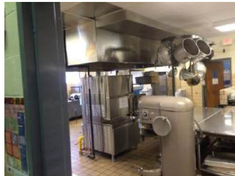
New kitchen equipment installed
