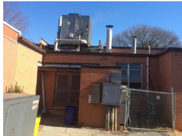
Roof top unit to be replaced
