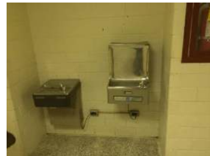
Water fountain fixtures to be replaced
