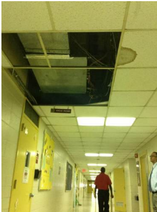
Hall Lighting to be Replaced
