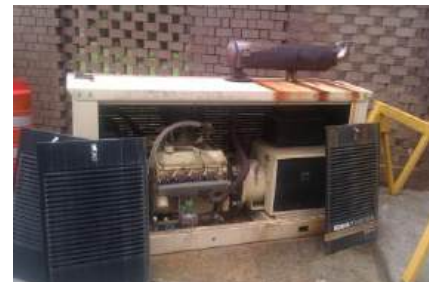
Bethune generator next to change
