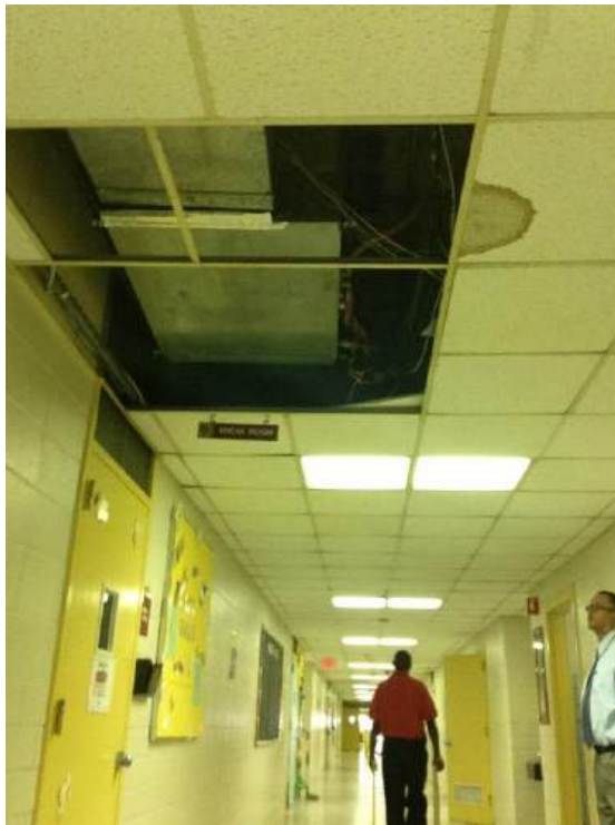
Hall Lighting to be Replaced
