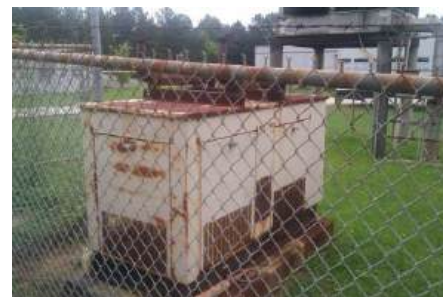
Old generator returned to DCSD
