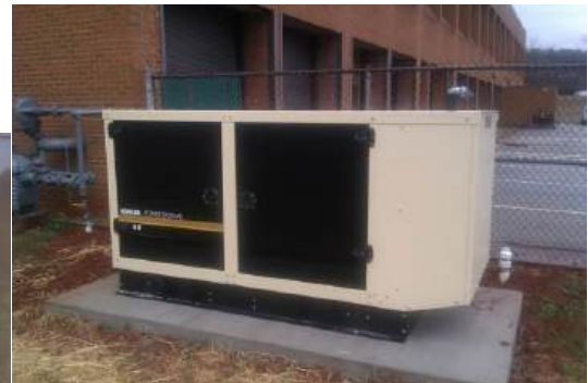
Emergency Generator for DHST-S
