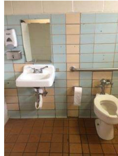
Bathroom fixtures to be replaced
