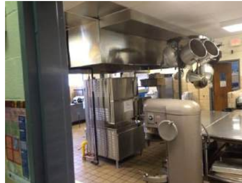
New kitchen equipment installed
