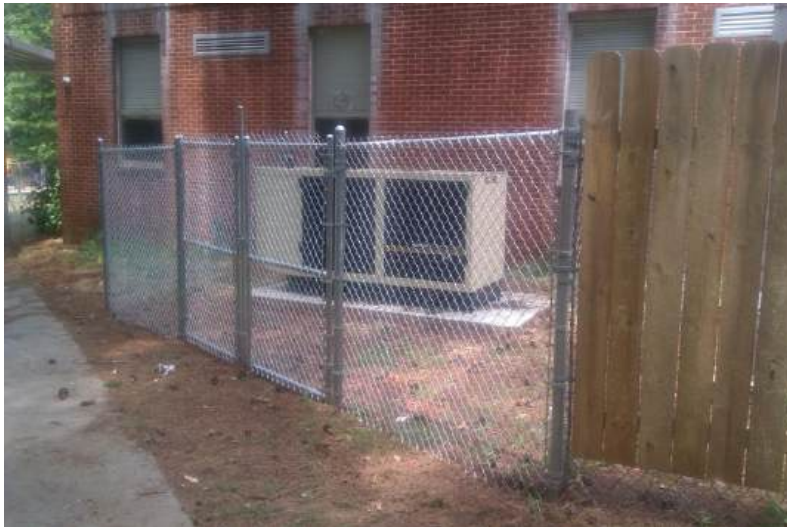
Emergency Generator for Chesnut ES
