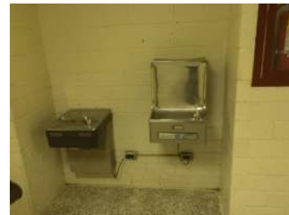
Water fountain fixtures to be replaced
