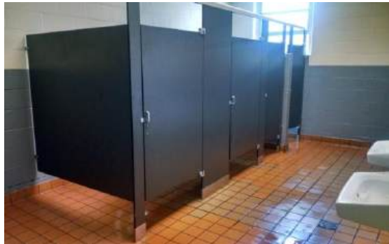
Chapel Hill ES Restroom after Construction
