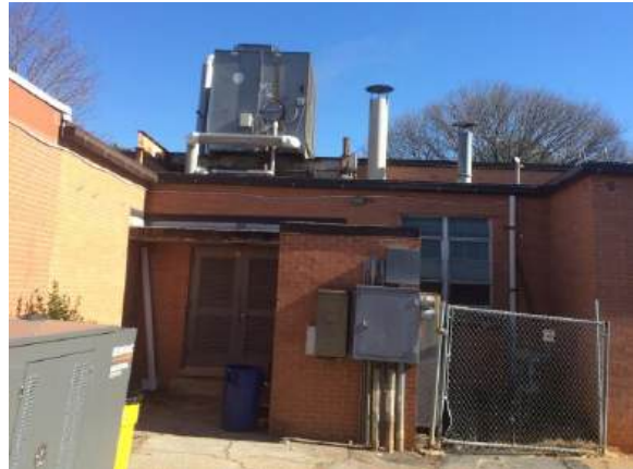
Roof top unit to be replaced
