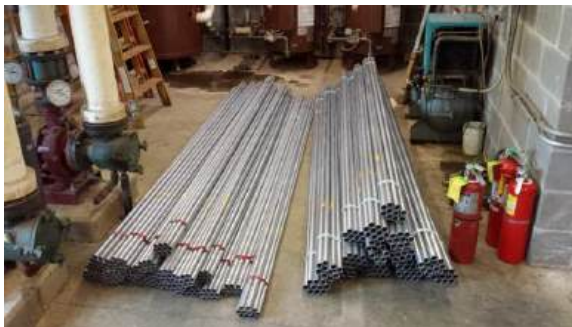
New electrical conduit ready for installation
