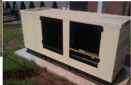
Emergency Generator for McNair MS
