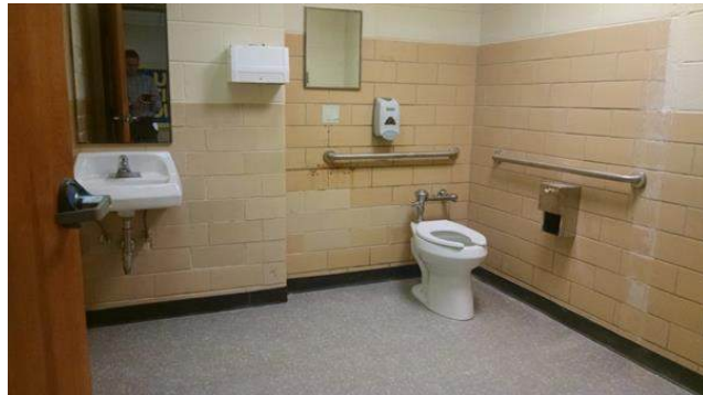
Chapel Hill ES Restroom after Construction
