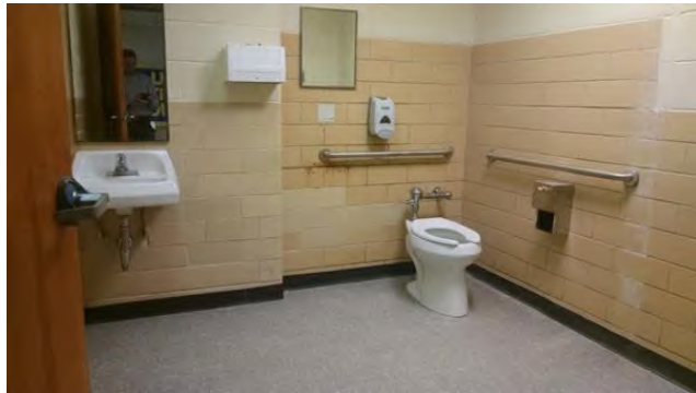
Chapel Hill ES Restroom after Construction
