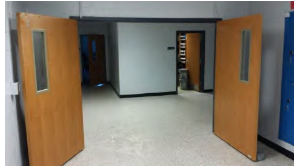
Corridor doors waiting on push bar openers
