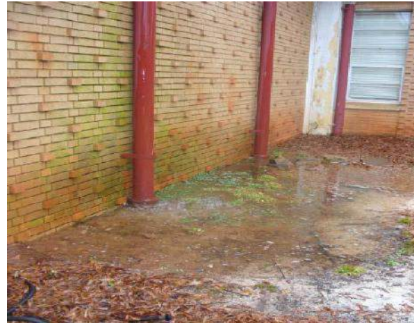
Improper drainage resulting in standing water
