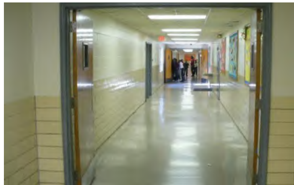
Existing fluorescent fixtures
