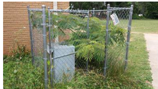
Gym transformer to be upgraded
