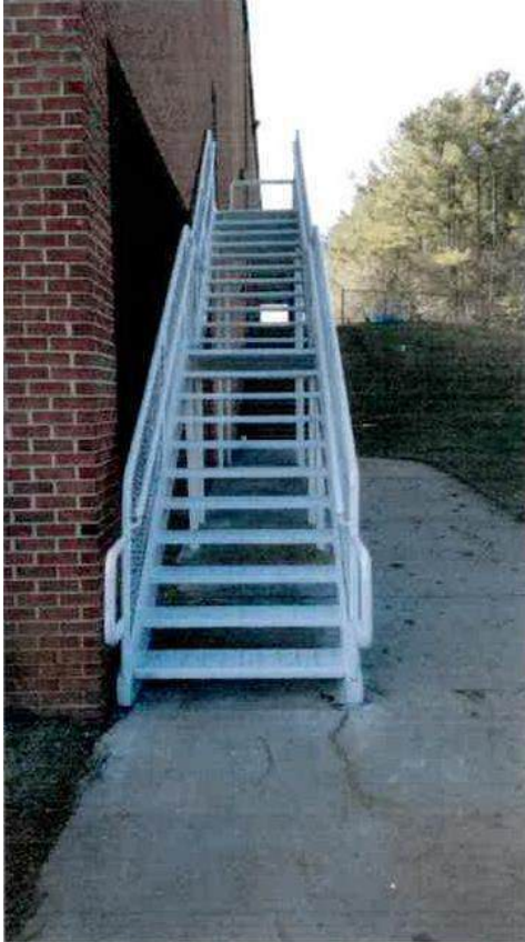
Metal Stairs over sanitary line to be reworked
