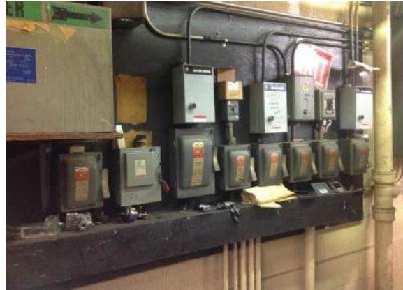
Electrical distribution system
