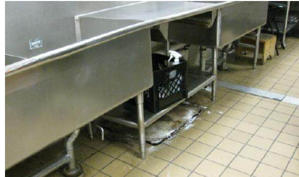
Existing under-sink grease trap
