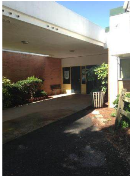
Sequoyah MS, Main Entrance Lacking ADA Access
