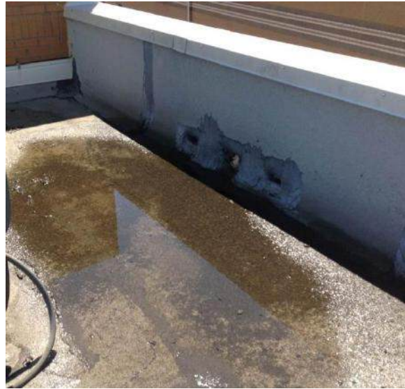
Ponding near the rooftop HVAC equipment
