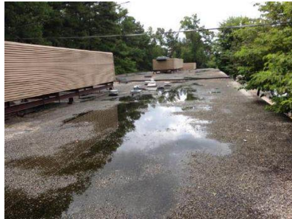
View of ponding water at the northwest roof area
