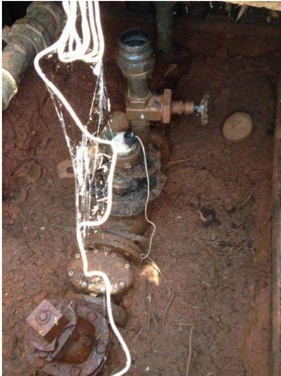
Backflow preventer to be replaced
