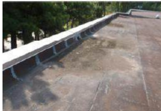
Roof shows signs of ponding water
