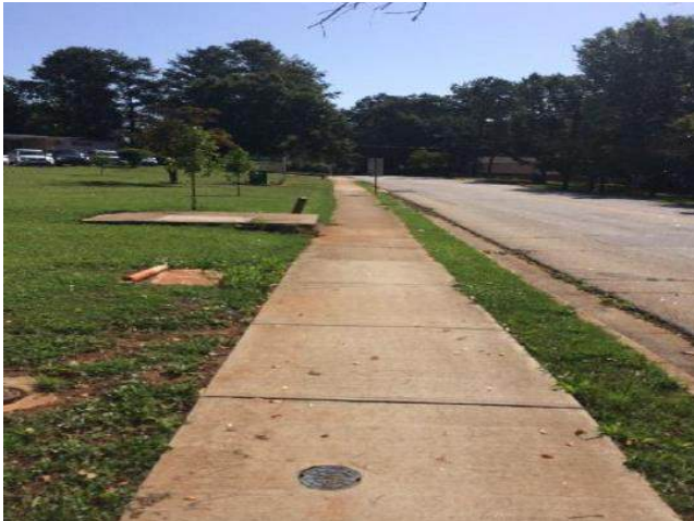
Backflow to be raised above ground
