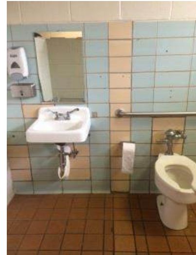
Bathroom fixtures to be replaced
