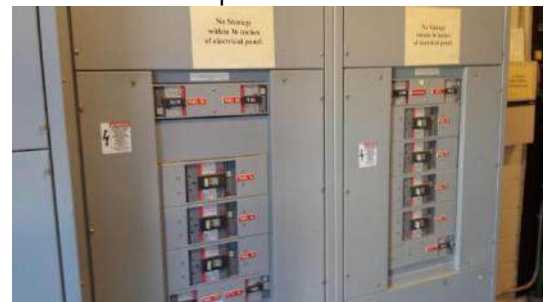
Main switchgear for Freedom MS
