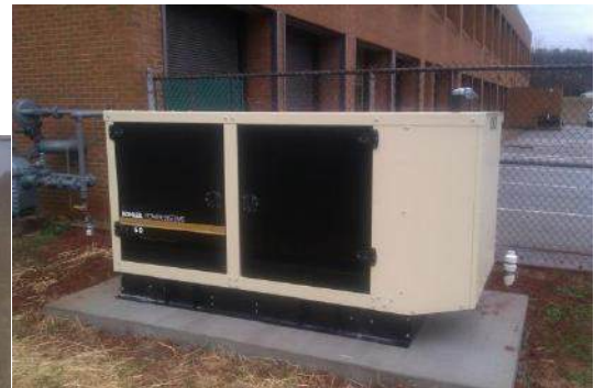
Emergency Generator for DHST-S
