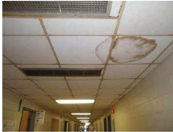
Stained ceiling tile
