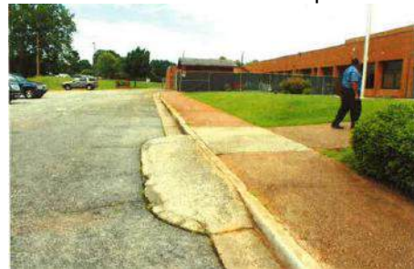
ADA ramp to be corrected
