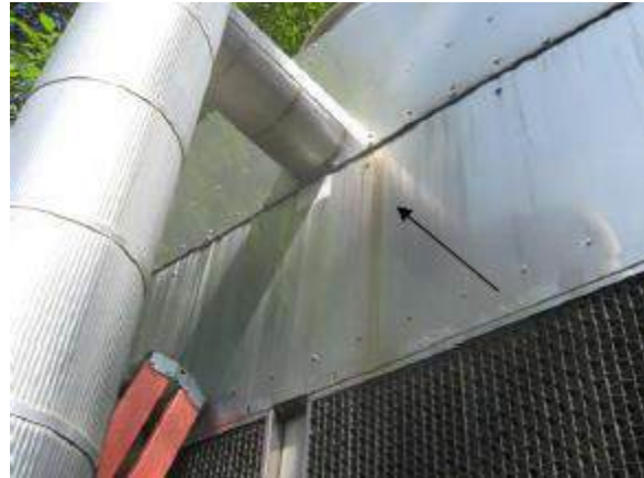
Cooling tower leak to be repaired
