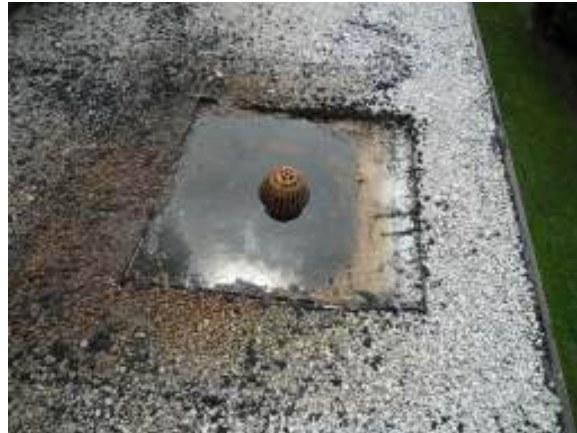
Clogged roof drain retaining water
