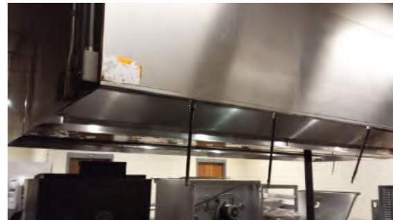
Kitchen hood scheduled for replacement
