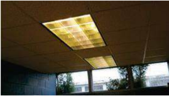
Existing lighting fixtures
