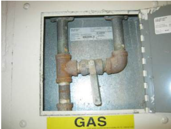
Typical valve box located in each of the 12 Science Lab rooms
