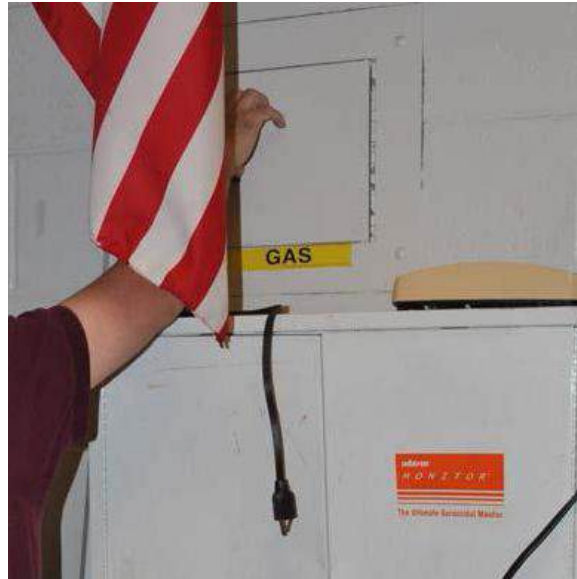
Emergency equipment shutoffs located above germicidal cabinets
