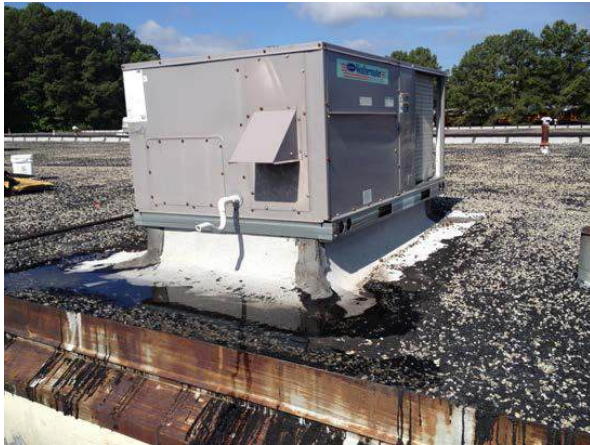
Ponding around roof HVAC unit
