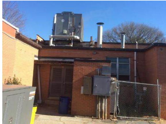
Roof top unit to be replaced
