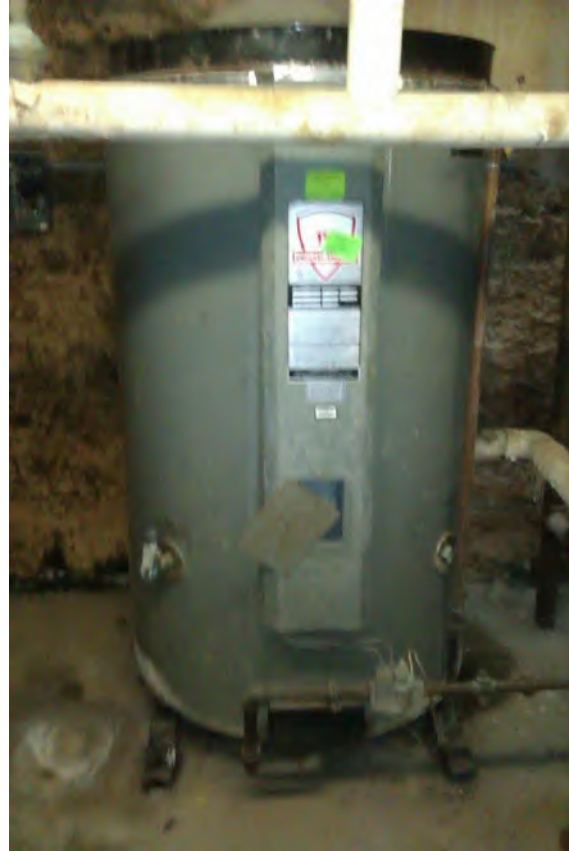
Gym water heater to be replaced
