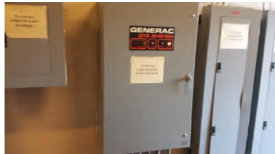
ATS to be replaced at Freedom MS
