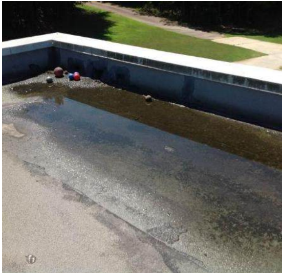
Ponding on the roof
