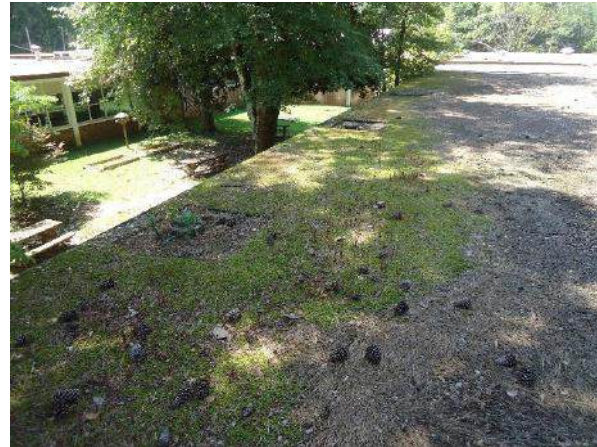
Vegetation growth over the surface of the roof system
