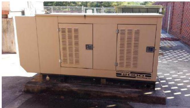
Generator to be replace and turned over to DCSD
