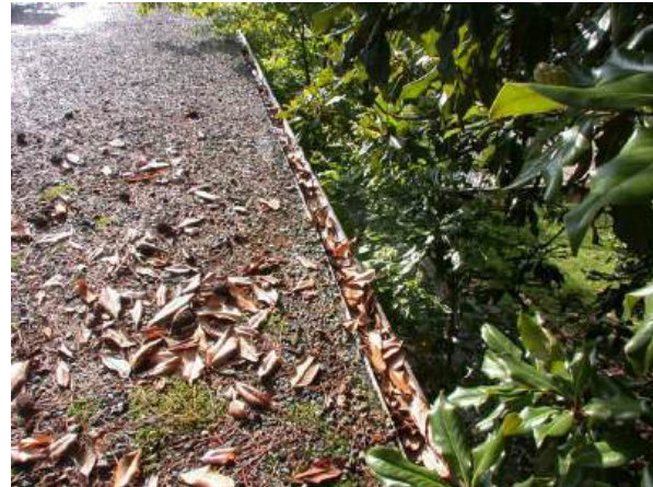
Area showing debris from trees and build-up on roof
