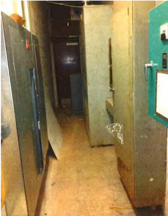
Existing problem with clearance
