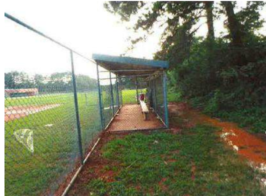
Baseball dugouts with water issues
