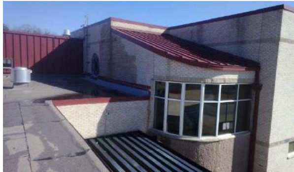
Roof to be repaired
