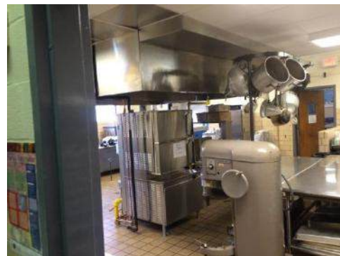
New kitchen equipment installed
