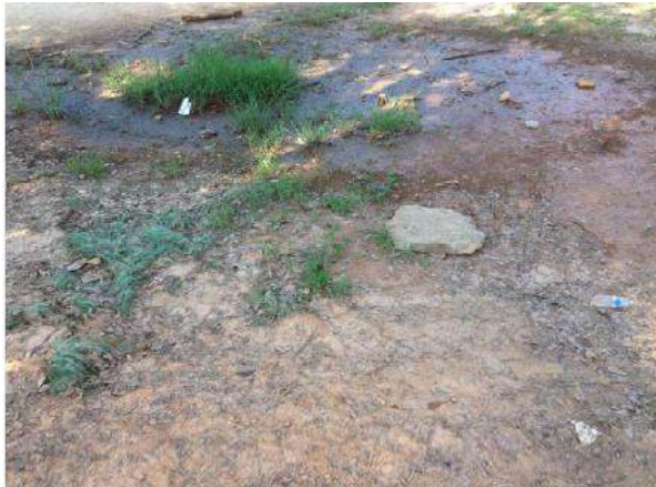
Ponding/Drainage/Erosion Issues at Playground
