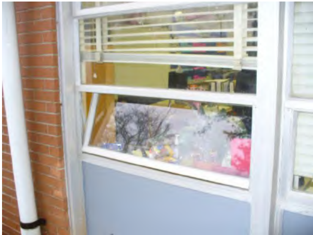
Inefficient single-pane existing windows
