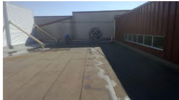
Roof to be repaired
