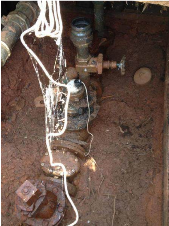
Backflow preventer to be replaced
