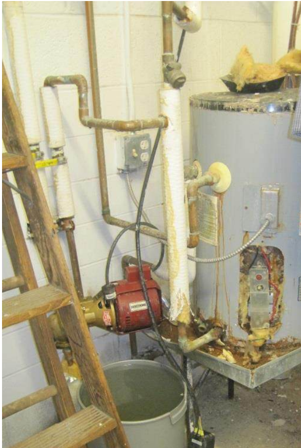
Existing damaged water heater
