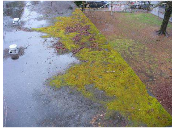
Vegetation overgrowth damaging the roof
