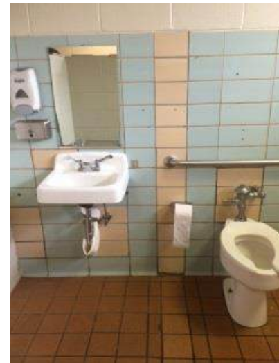
Bathroom fixtures to be replaced
