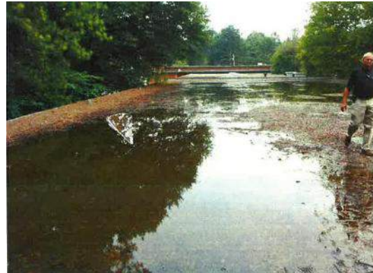
Ponding water on roofs
