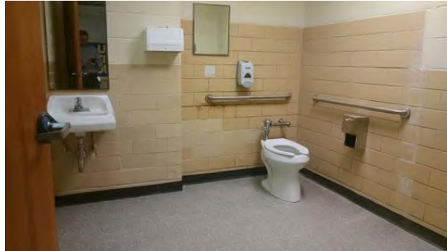
Chapel Hill ES Restroom after Construction
