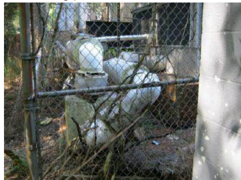
Cooling tower to be replaced
