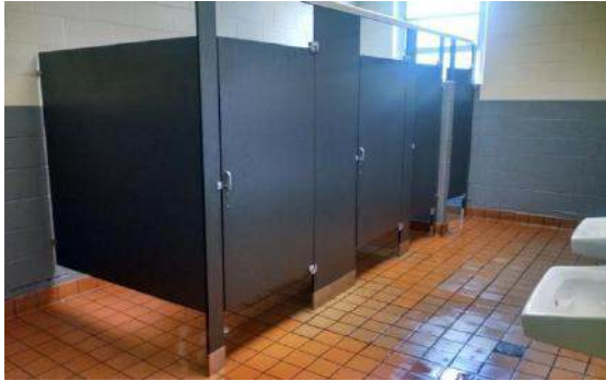
Chapel Hill ES Restroom after Construction
