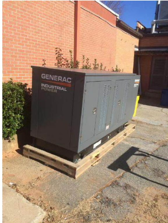
Emergency Generator to be installed
