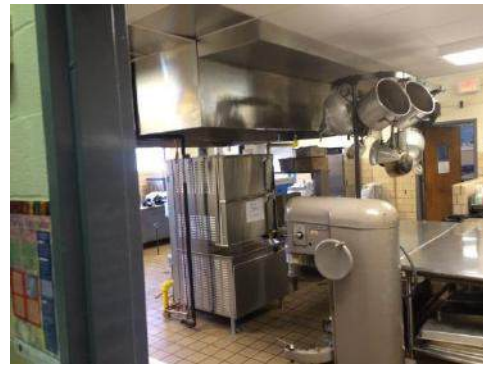
New kitchen equipment installed
