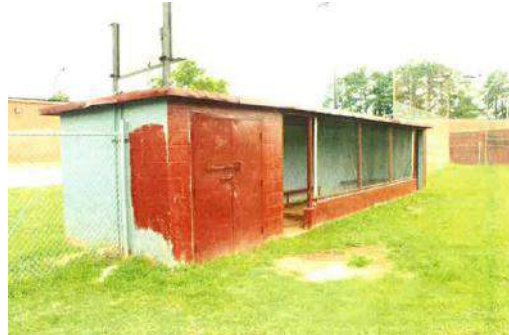
Baseball dugouts that need repairs
