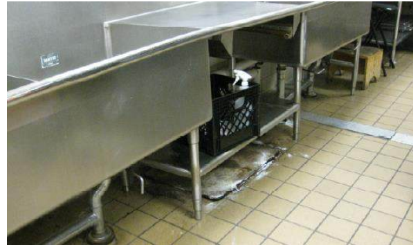
Existing under-sink grease trap
