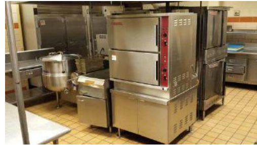
Kitchen equipment under review
