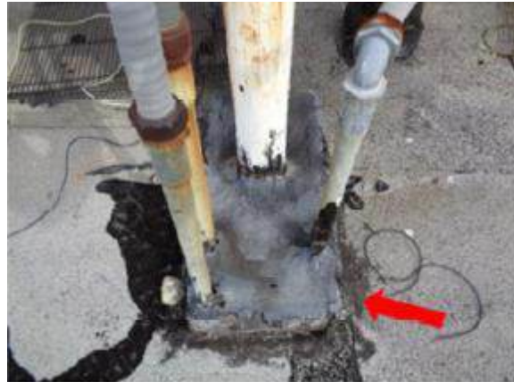
View of typical mechanical lines penetration curb/pitch pan condition on the main building roofs.
