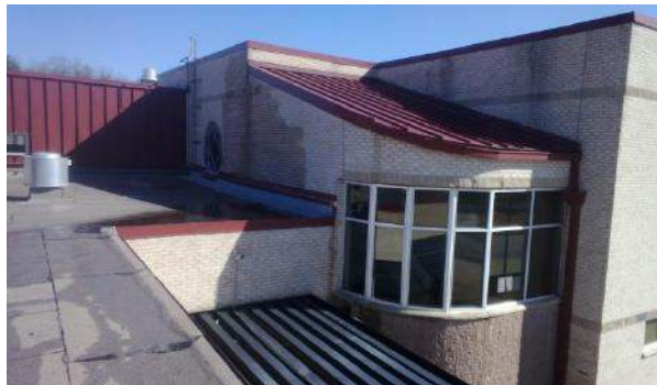
Roof to be repaired
