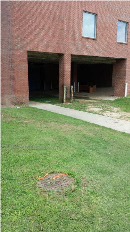
Sanitary line from manhole to be reworked
