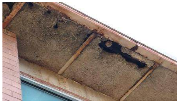
Tectum roof deck panels needing replaced
