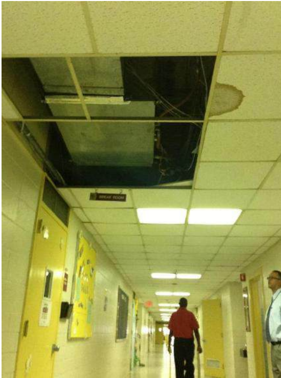
Hall Lighting to be Replaced
