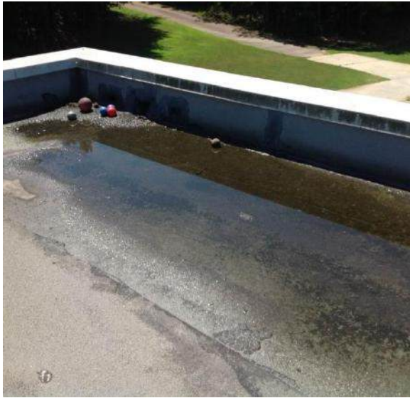
Ponding on the roof
