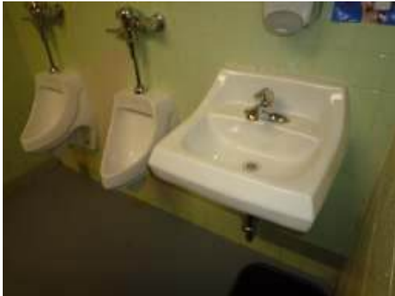
Existing mixture of new and old fixtures throughout the restrooms
