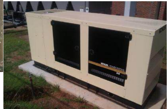
Emergency Generator for McNair MS
