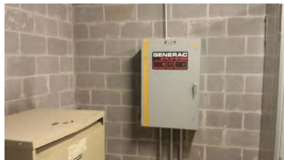
ATS to be replaced at Browns Mill ES
