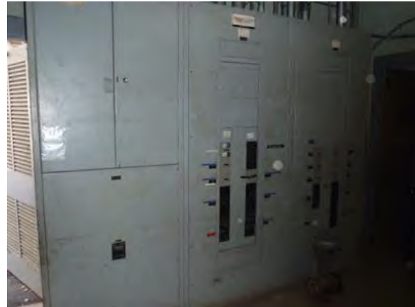
Electrical service entrance
