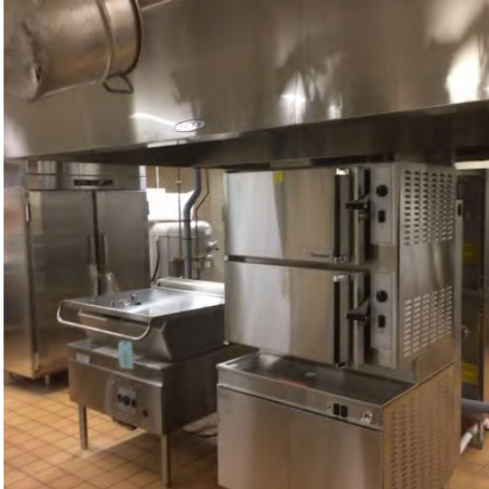
New Kitchen Equipment installed in the kitchen
