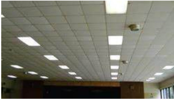
Existing lighting fixtures
