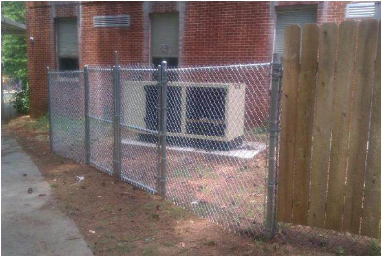
Emergency Generator for Chesnut ES
