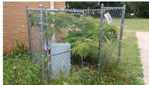
Gym transformer to be upgraded
