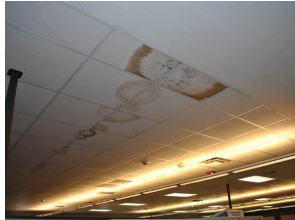
Interior ceiling tile damage from roof leaks
