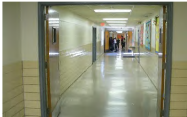
Existing fluorescent fixtures
