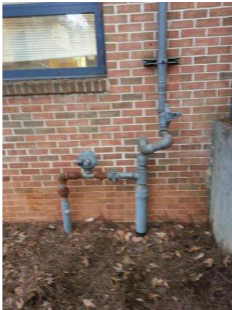
Montclair ES Gas service entrance
