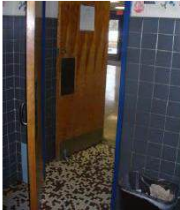
Restroom access configuration does not comply with ADA
