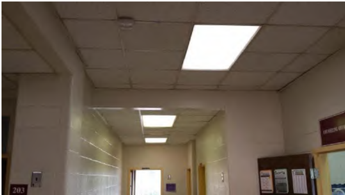
Corridors waiting on lighting change out
