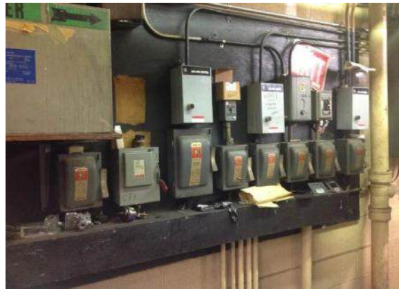
Electrical distribution system
