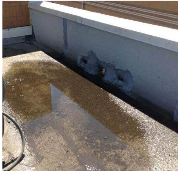
Ponding near the rooftop HVAC equipment
