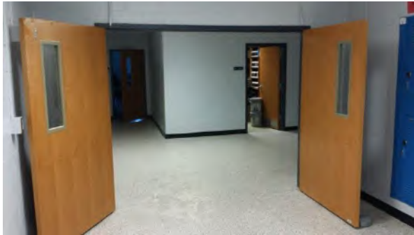
Corridor doors waiting on push bar openers
