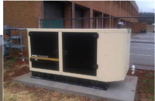
Emergency Generator for DHST-S
