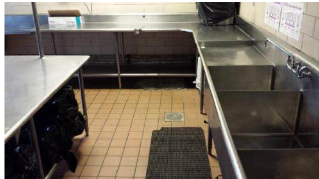
Kitchen grease trap be replaced
