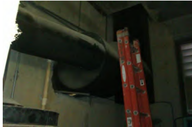
water heater exhaust duct to be adapted
