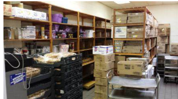
Kitchen dry storage shelvs needing replacement
