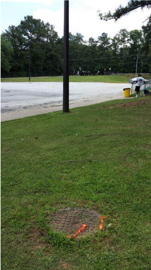
Sanitary lines to be reworked
