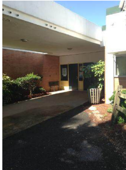
Sequoyah MS, Main Entrance Lacking ADA Access
