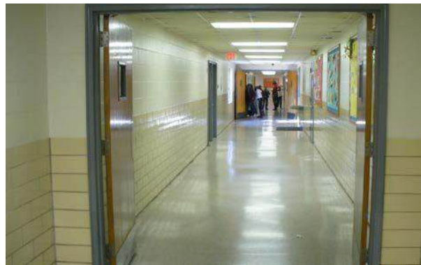
Existing fluorescent fixtures
