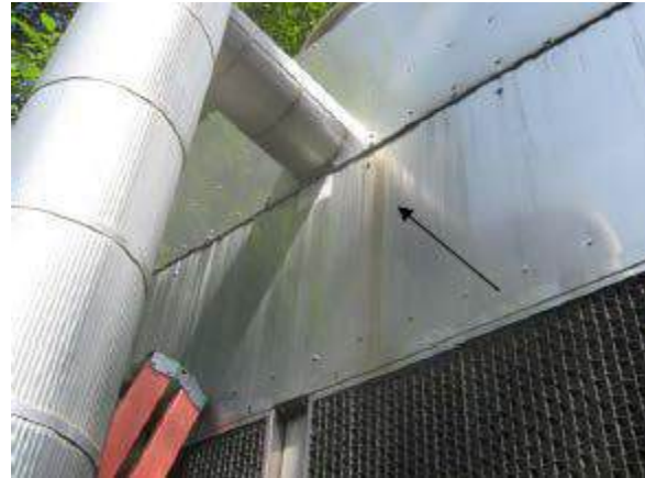
Cooling tower leak to be repaired
