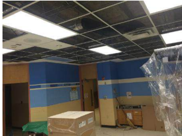
Classroom: New HVAC, Ceiling Grid to be Installed, and Lighting to be Replaced
