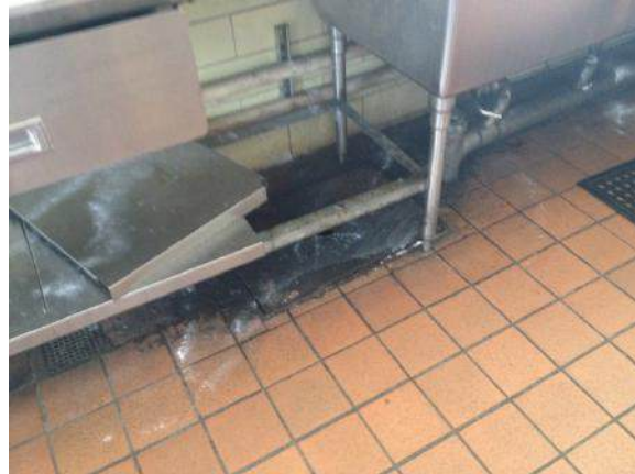
Grease trap to be replaced
