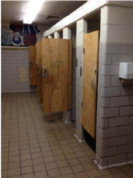
Existing student restroom needs ADA upgrades
