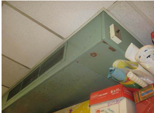
Typical HVAC unit serving classroom to be upgraded
