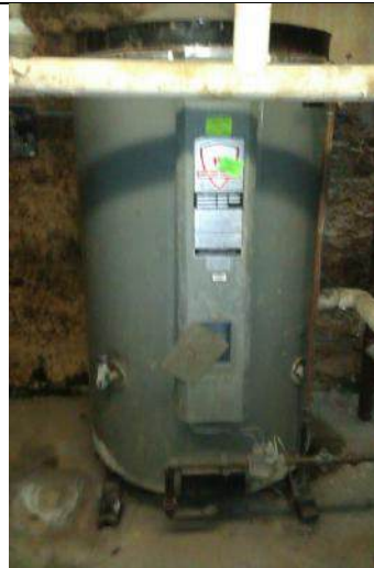
Water heater to be replaced
