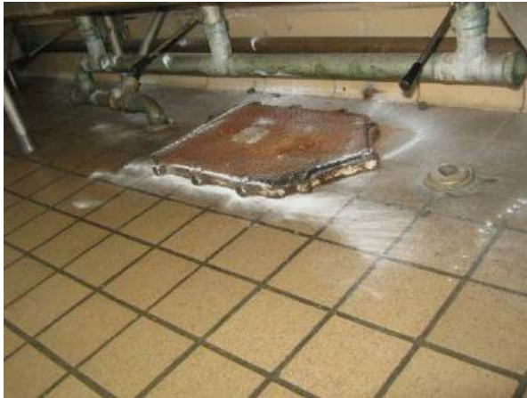
Existing grease trap
