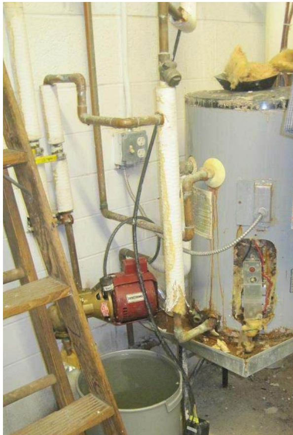
Existing damaged water heater
