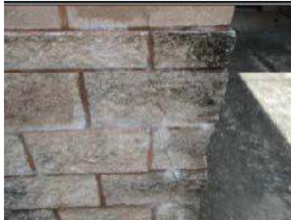
Exterior veneer at the exterior corner of Room 615 formed vertical cracks
