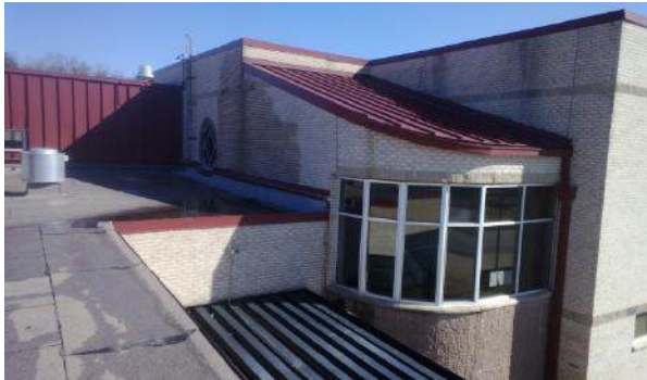
Roof to be repaired
