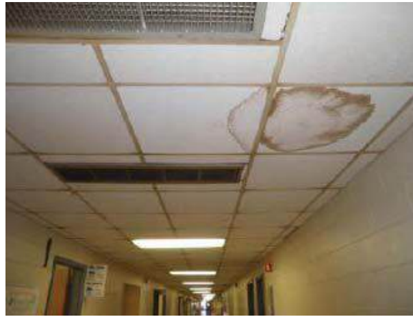
Stained ceiling tile
