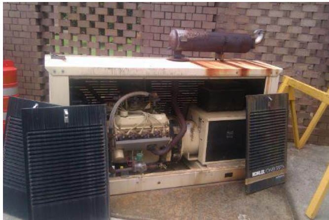
Current Mary Mcload Bethune MS emergency generator
