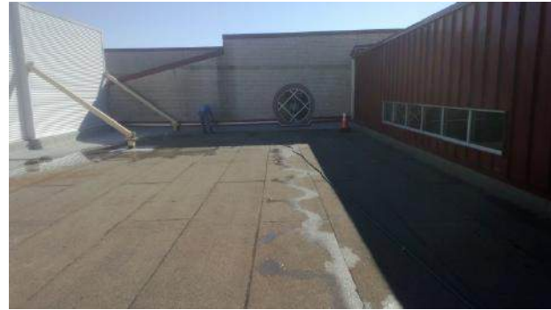
Roof to be repaired
