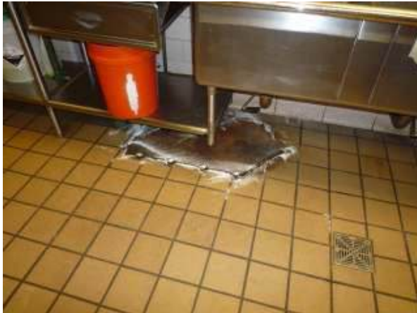
Existing interior grease trap
