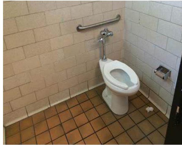
Existing handicap stall in girls' restroom
