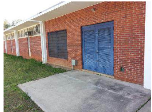
Huntley Hills ES possible generator location
