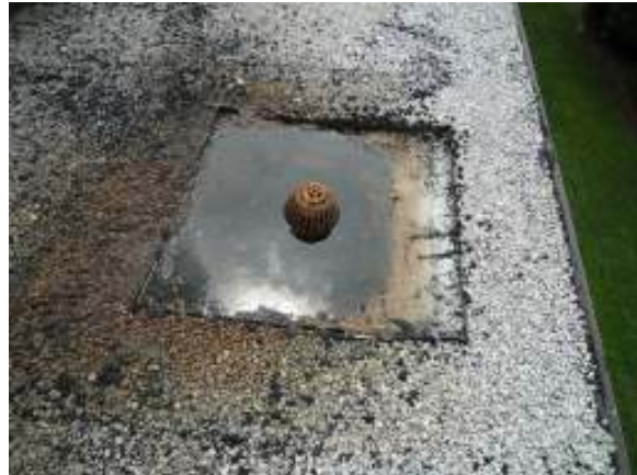
Clogged roof drain retaining water
