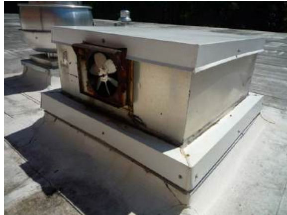
Roof work to be done
