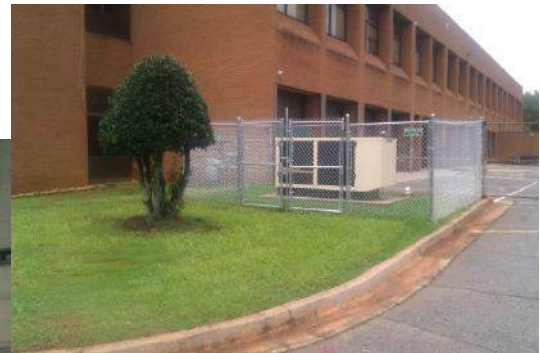
Emergency Generator for DHST-S
