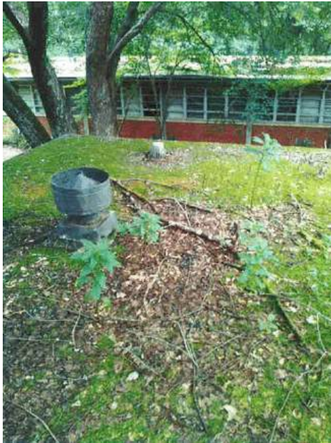
Organic material covering roofing
