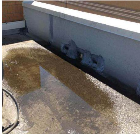
Ponding near the rooftop HVAC equipment
