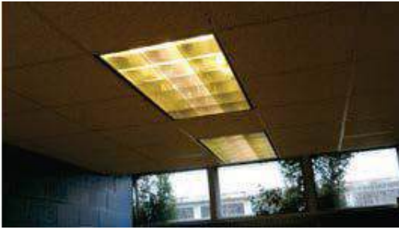
Existing lighting fixtures
