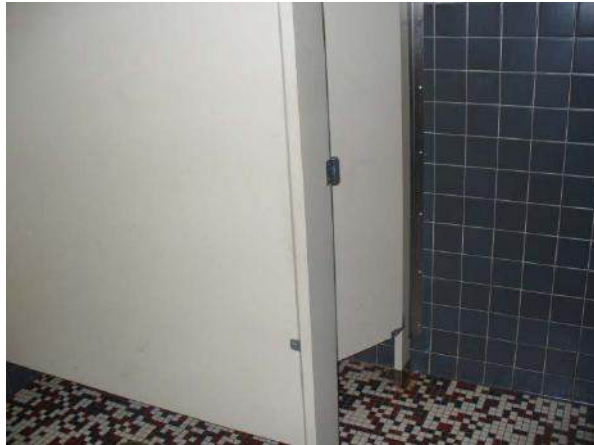
Boys restroom stall does not comply w/ ADA (5')
