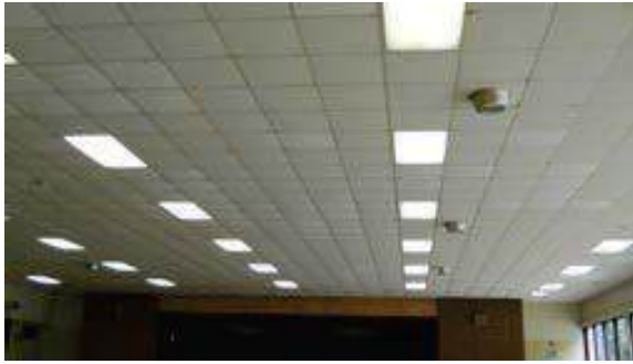
Existing lighting fixtures
