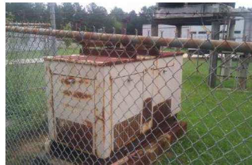
Current generator at Browns Mill ES
