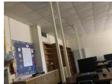
Classroom Lighting to be Replaced
