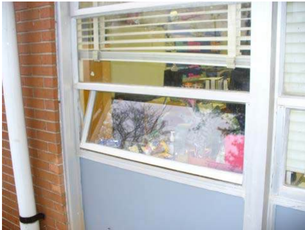
Inefficient single-pane existing windows
