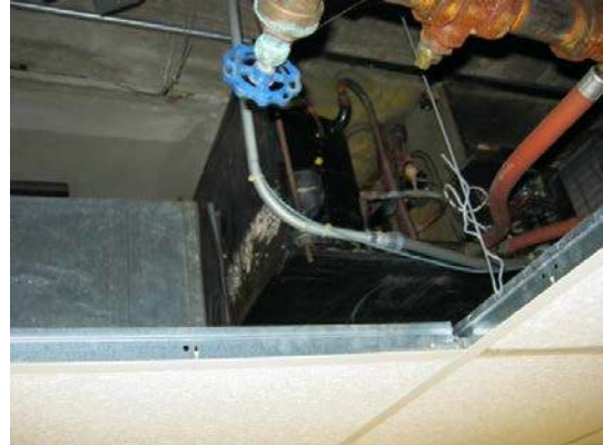
Heat pumps scheduled for replacement
