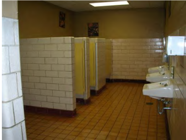
Typical example of CMU walls, high grab bars, and corroded plumbing access panel
