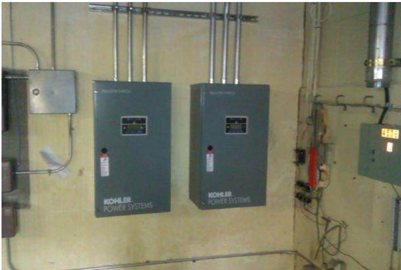
New ATS controllers for Chesnut ES
