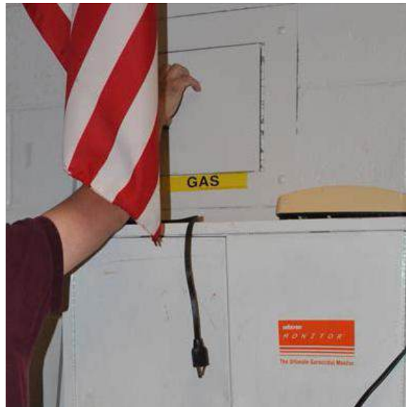
Emergency equipment shutoffs located above germicidal cabinets
