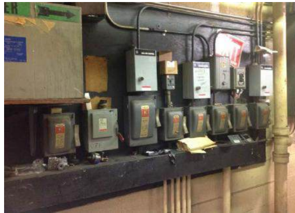
Electrical distribution system
