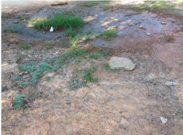
Ponding/Drainage/Erosion Issues at Playground
