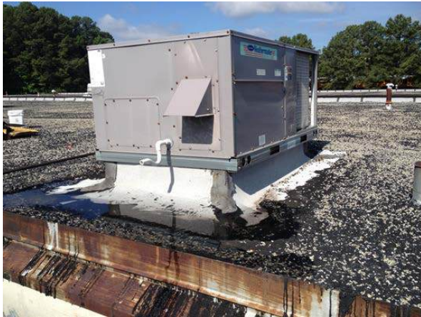
Ponding around roof HVAC unit
