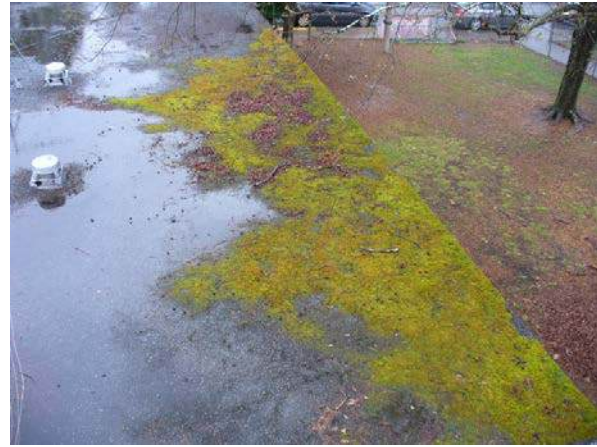
Vegetation overgrowth damaging the roof
