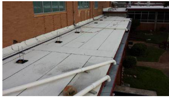
PVC pipes to bring water from the Gym roof
