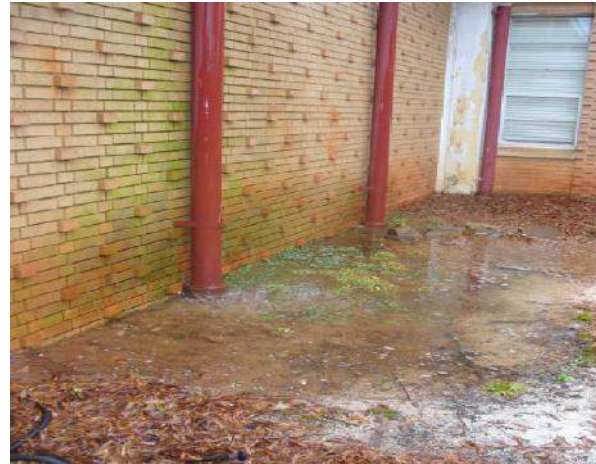
Improper drainage resulting in standing water
