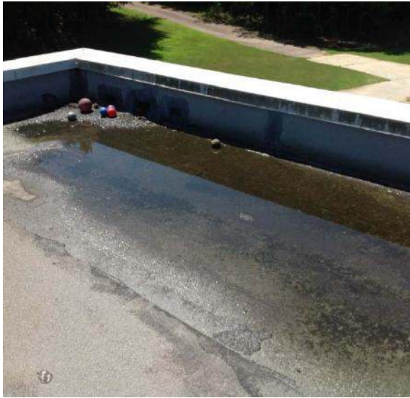
Ponding on the roof
