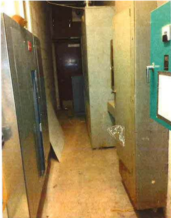
Existing problem with clearance
