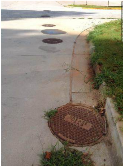
Existing grease trap
