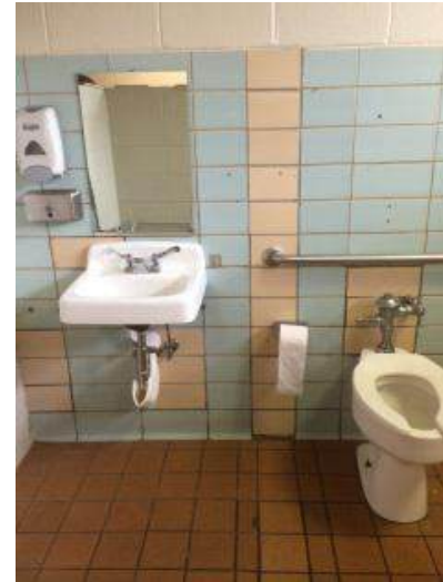
Bathroom fixtures to be replaced
