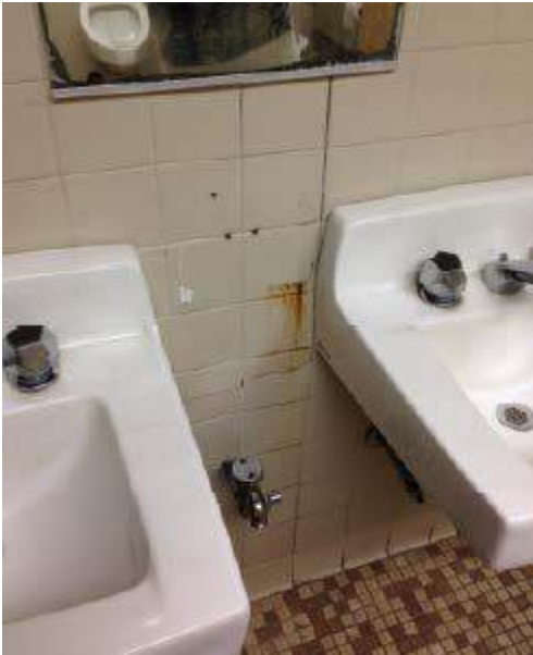
Typical tile wall damage and non ADA compliant sink knobs
