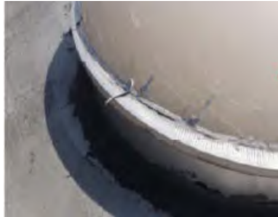
Plastic domes of the skylights deteriorated and cracked
