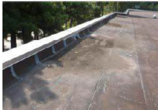
Roof shows signs of ponding water
