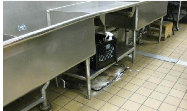
Existing under-sink grease trap
