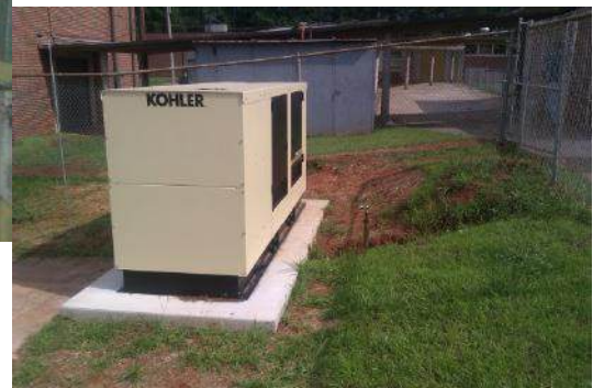
Emergency Generator for McNair MS
