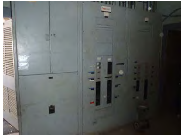
Electrical service entrance
