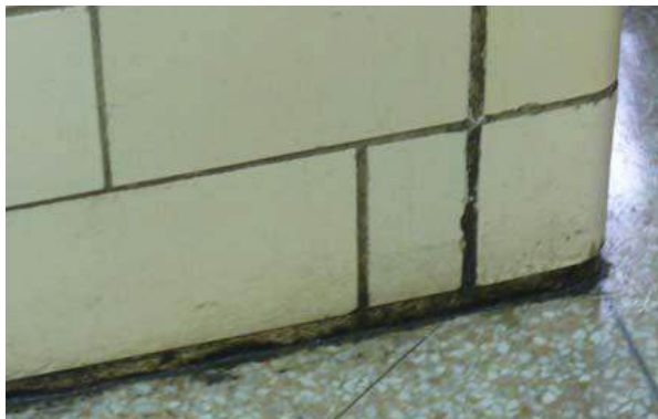
Existing glazed block with no wall base
