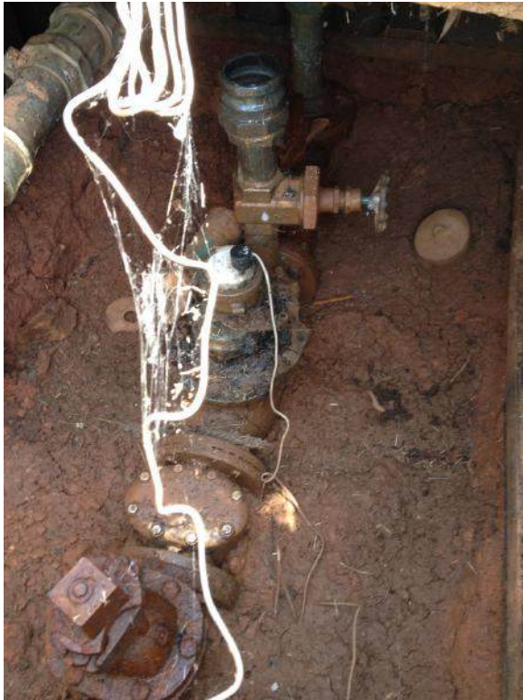
Backflow preventer to be replaced
