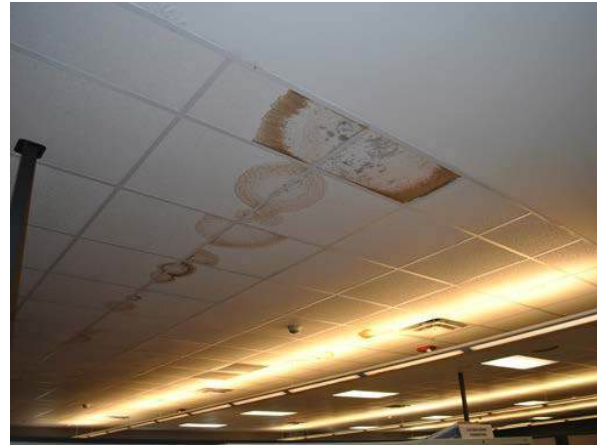
Interior ceiling tile damage from roof leaks
