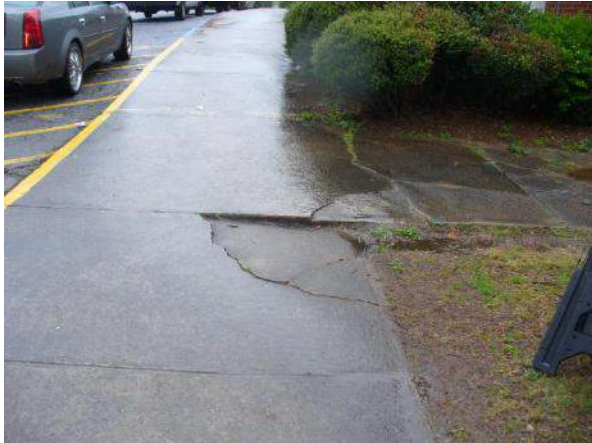
Replacement of pedestrian paving needed
