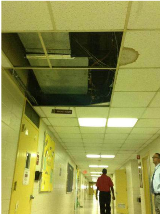
Hall Lighting to be Replaced
