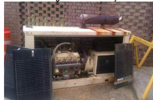
Current generator at Bethune MS
