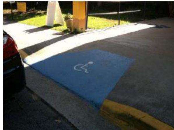
Curb ramp does not comply with ADA
