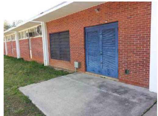
Huntley Hills ES possible generator location
