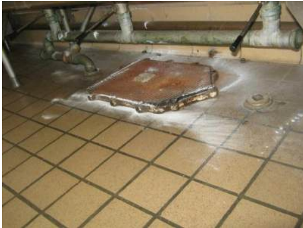
Existing grease trap
