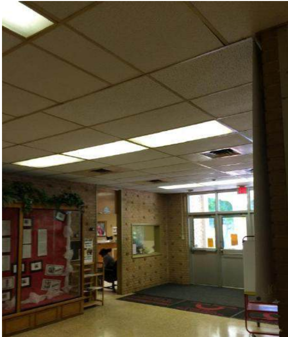
Main Corridor: New HVAC, Ceiling Grid to be Installed, and Lighting to be Replaced
