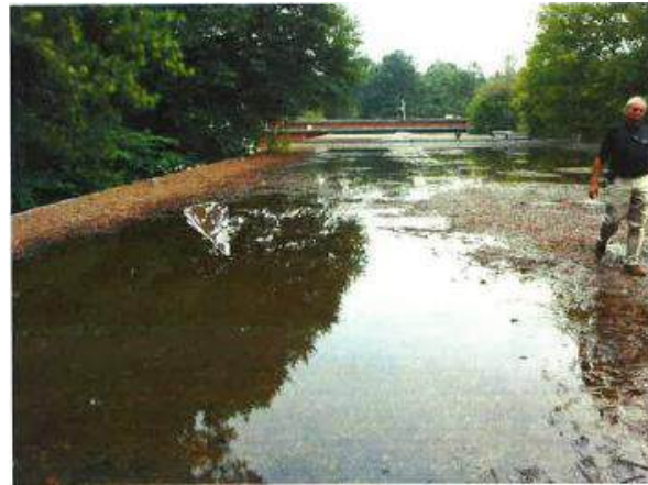
Existing roof with significant ponding of rain water
