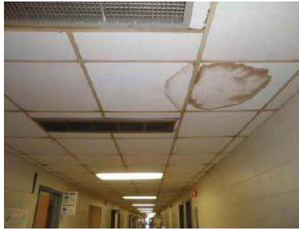
Stained ceiling tile
