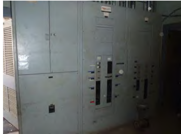
Electrical service entrance
