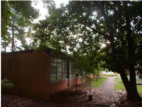
Trees contacting building elements, particularly gutters and roof
