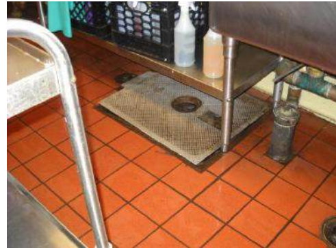
Kitchen grease trap
