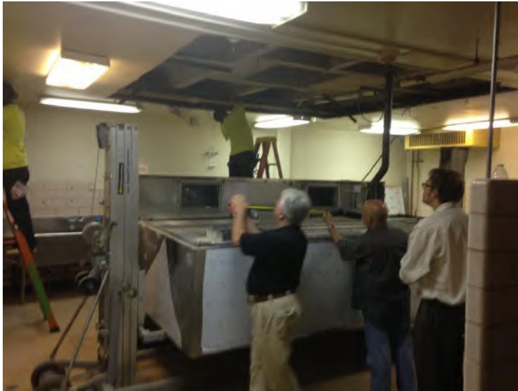
Phase 5 Construction: New Kitchen hood, HVAC, Ceiling Grid to be Installed, Tile and Lighting to be Replaced
