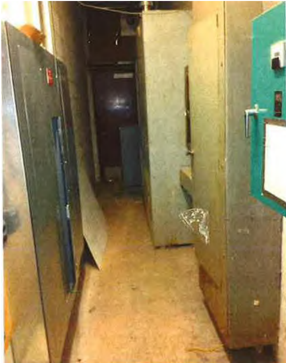
Existing problem with clearance
