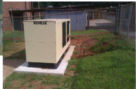
Emergency Generator for McNair MS
