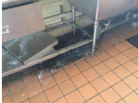
Grease trap to be replaced
