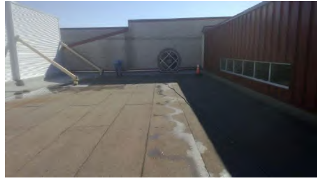
Roof to be repaired
