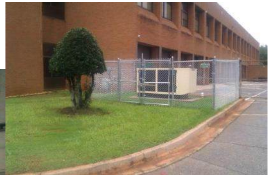
Emergency Generator for DHST-S
