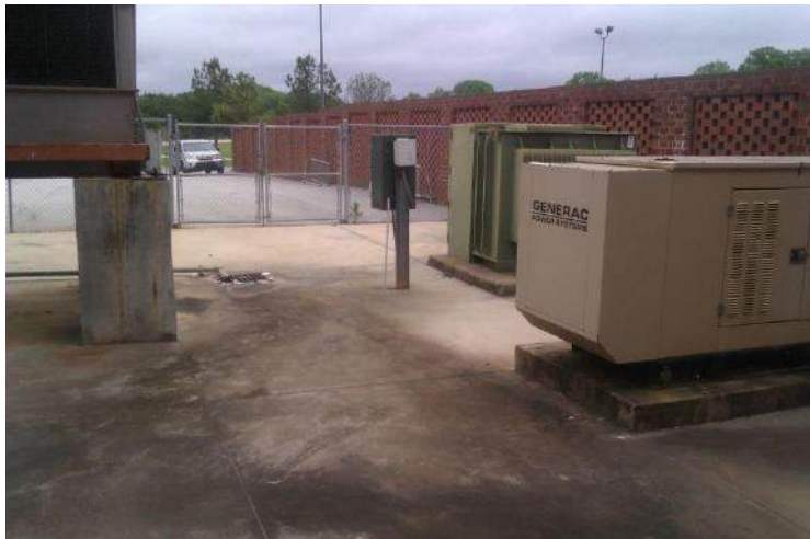
Current Freedom MS emergency generator
