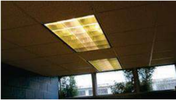
Existing lighting fixtures
