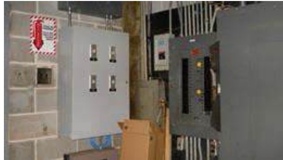
Electrical service and distribution equipment is aged beyond service life
