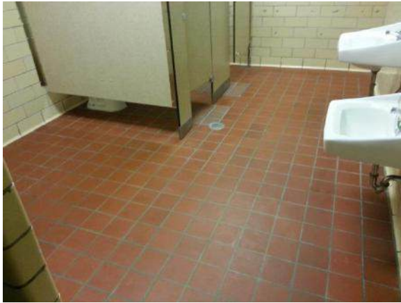
Ashford Park ES student restroom toilet partitions
