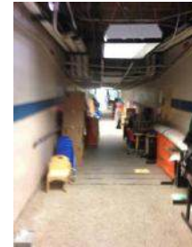
Phase 5: Corridor: New HVAC, Ceiling Grid to be Installed, Tile and Lighting to be Replaced
