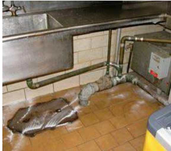
Existing grease trap
