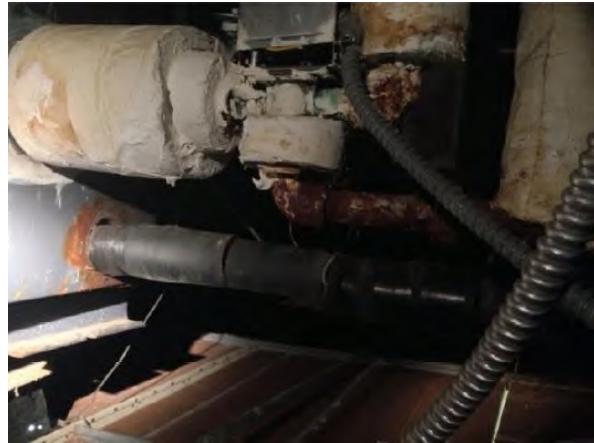
Media Center air handling unit is not operational
