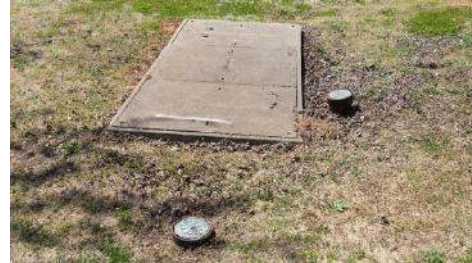
Backflow to be raised out of vault
