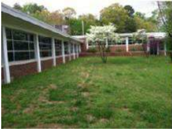
Courtyard at Bldg. #100 has had numerous blockages
