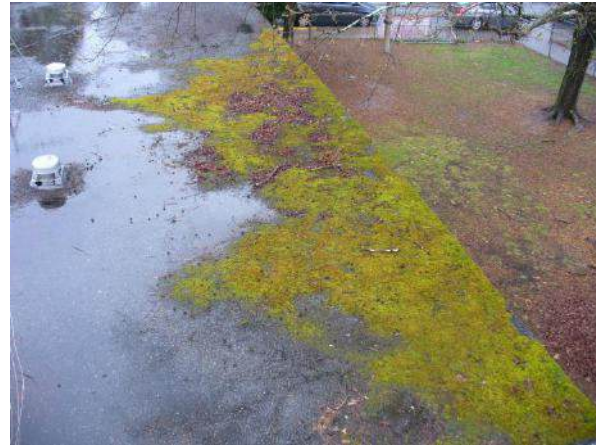
Vegetation overgrowth damaging the roof
