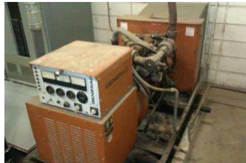
Generator scheduled for replacement
