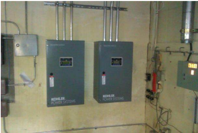
New ATS controllers for Chesnut ES
