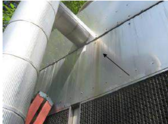
Cooling tower leak to be repaired
