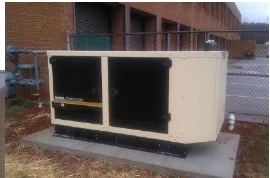
Emergency Generator for DHST-S
