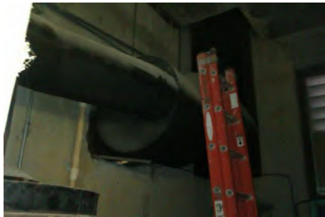
Water heater exhaust ductwork
