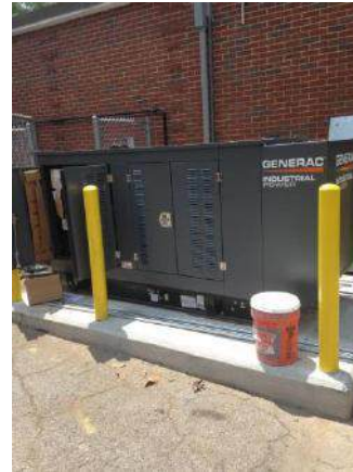
Installation of new emergency generator tested and approved by DeKalb Fire Marshal
