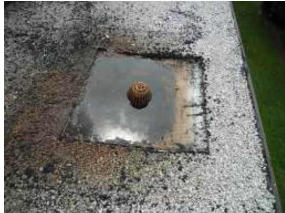
Clogged roof drain retaining water
