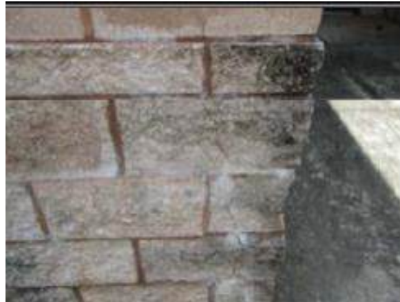
Exterior veneer at the exterior corner of Room 615 and several locations under the windows have formed vertical cracks
