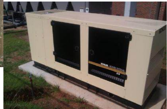
Emergency Generator for McNair MS
