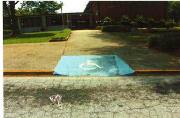
Existing handicap curb cut does not comply with ADA
