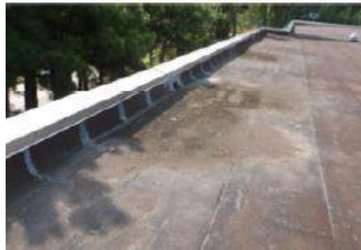
Roof shows signs of ponding water
