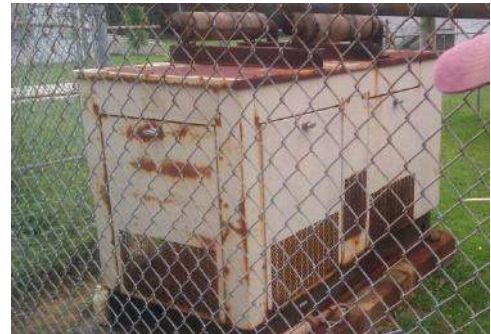
Current Browns Mill ES generator
