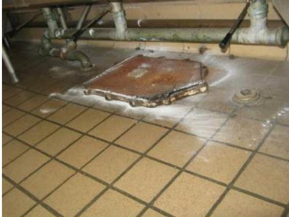
Existing grease trap
