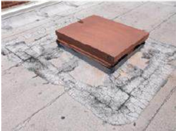
View of alligator cracking along the roof membrane and flashing at an access hatch on the low gymnasium roof area
