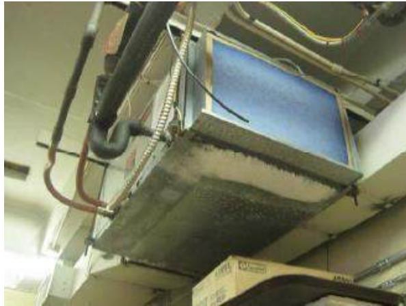
Ice Formed On Malfunctioning Unit in Kitchen Dry Storage Area
