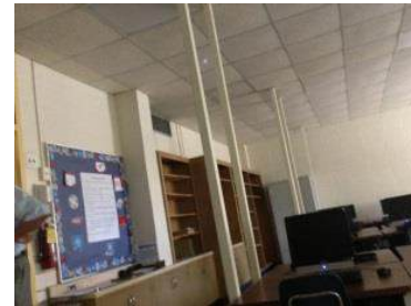
Classroom Lighting to be Replaced
