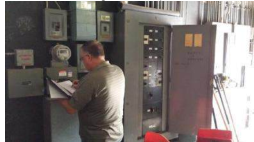
Power study for new equipment
