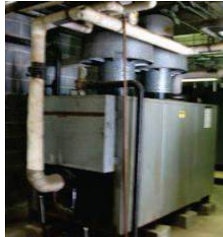
Existing heating hot water system not functioning
