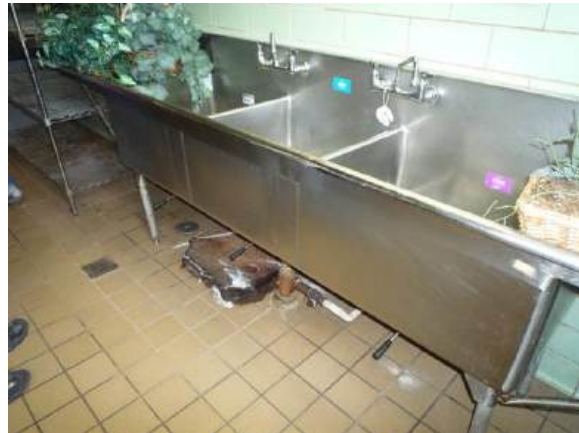
Existing interior grease trap
