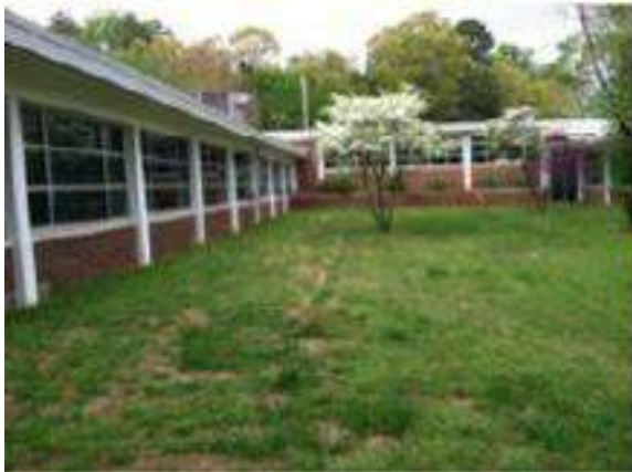
Courtyard at Bldg #100 has had numerous blockages
