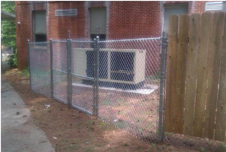
Emergency Generator for Chesnut ES
