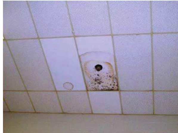
Building systems and finishes impacted by leaks and water infiltration
