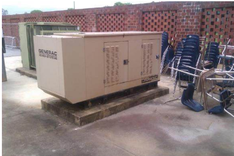
Current Freedom MS emergency generator
