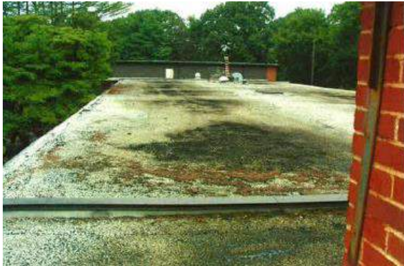
Existing roof showing signs of ponding water
