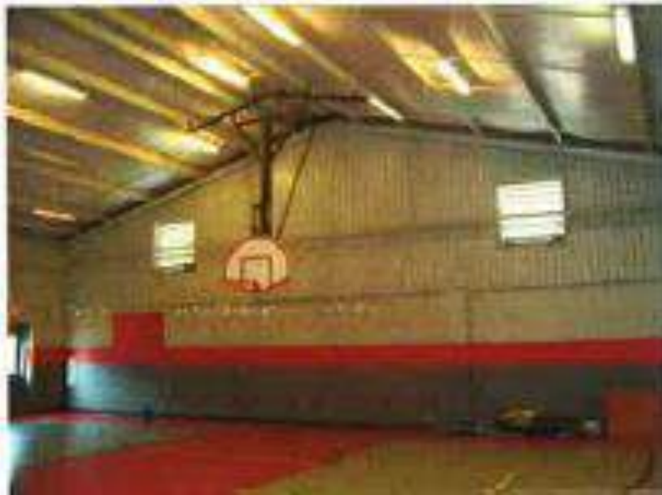
Existing gymnasium exhaust fan and louvers no longer function
