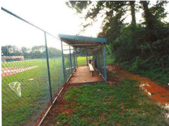
Softball dugout, showing standing storm water behind dugout
