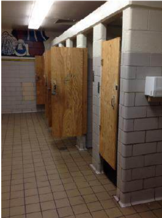
Existing student restroom needs ADA upgrades
