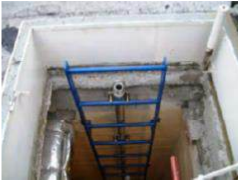
Existing roof hatch is not up to code
