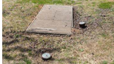
Backflow to be raised out of vault
