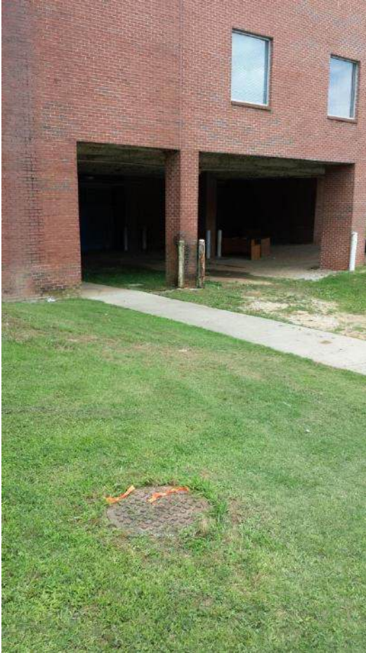
Sanitary lines to be reworked
