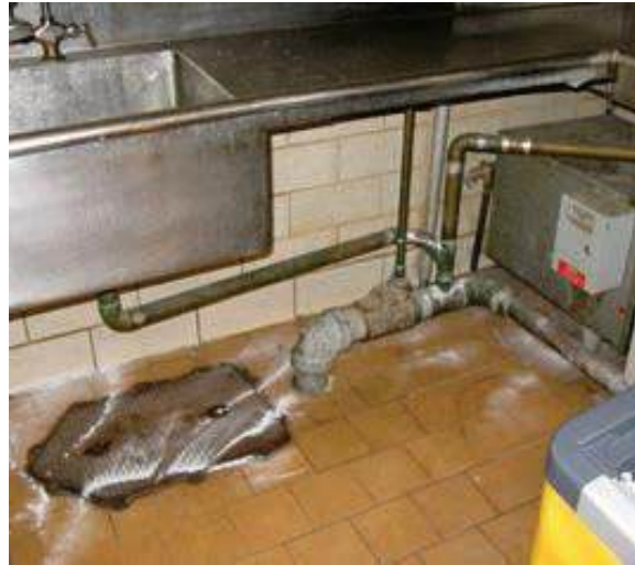
Existing grease trap
