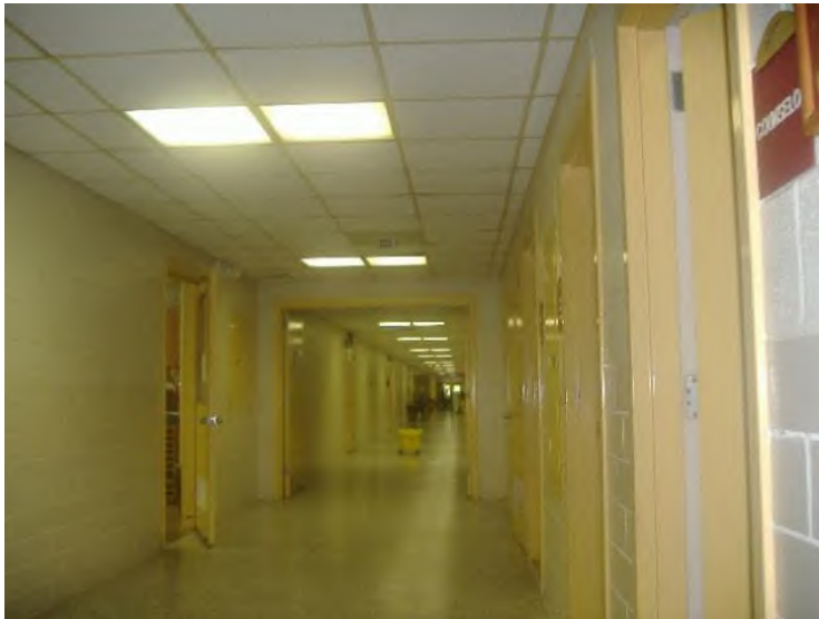
Corridor ceiling and lighting fixtures to be replaced
