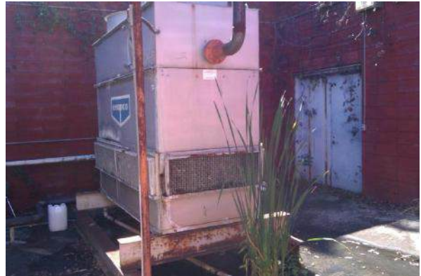
Cooling tower in back mechanical yard
