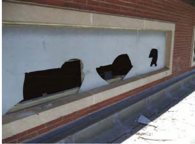
Transite panels at Sky Haven ES
