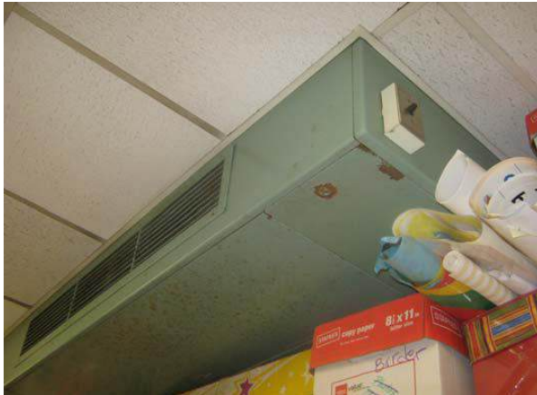
Typical HVAC unit serving classroom (not functioning at time of site visit)
