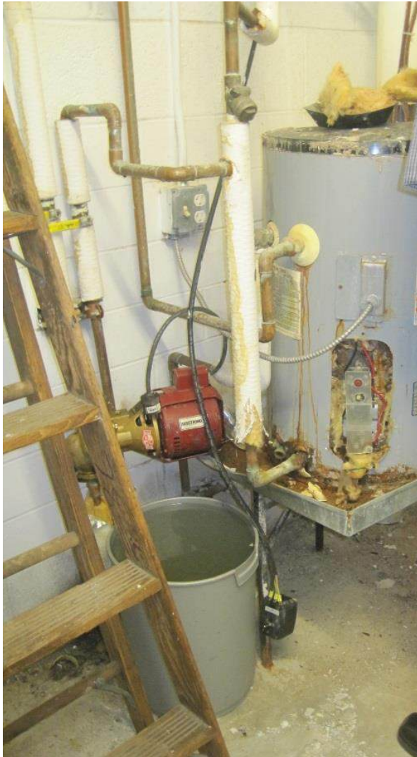
Existing damaged water heater
