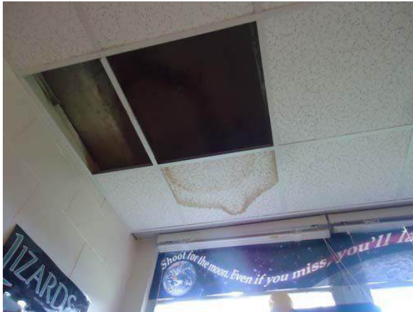
Signs of roof leakage into a classroom area
