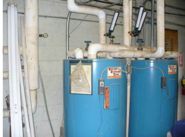
Water storage tanks to be replaced with gas fired water heater
