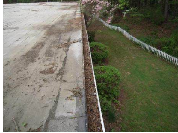
View of organic roof debris which has clogged the gutters at the north building wing
