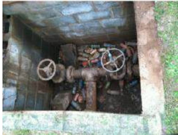
Water service vault with isolation gate valves between building #100 and #200
