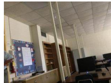
Classroom Lighting to be Replaced
