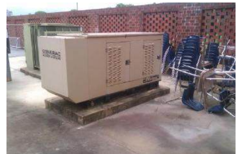
Existing Generator for Freedom MS
