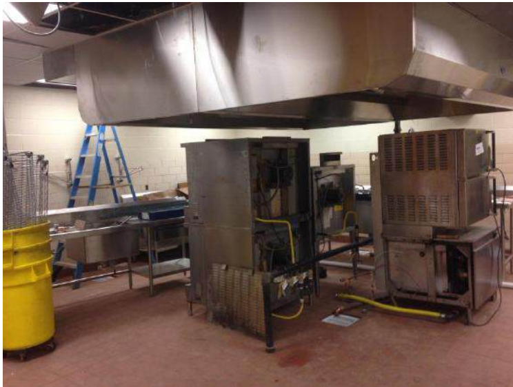
New Kitchen Floor Tile Over Terrazzo was Installed, New Hood, HVAC, Ceiling Grid was Installed, Tile and Lighting was Replaced
