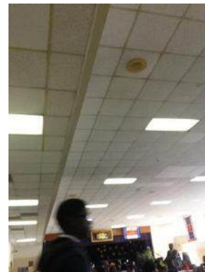
Cafeteria Ceiling Grid Covers to be Installed, Tile and Lighting to be Replaced
