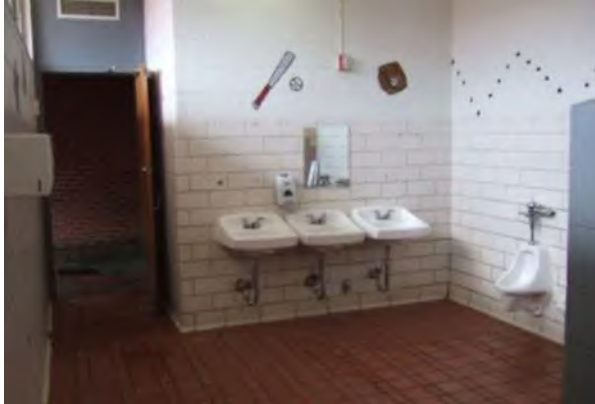
Midway ES Existing Bathroom
