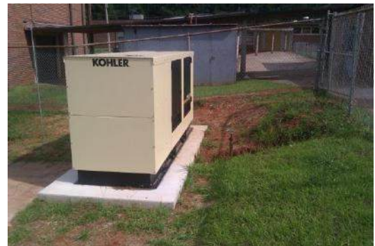
New Generator at McNair MS
