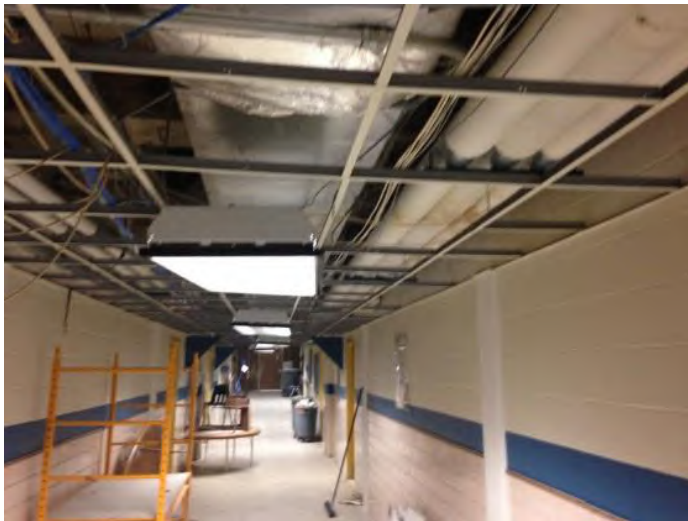
Phase 3 Construction: Main Corridor : New HVAC, Ceiling Grid to be Installed, Tile and Lighting to be Replaced
