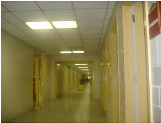
Corridor: New HVAC, Ceiling Grid to be Installed, Tile and Lighting to be Replaced
