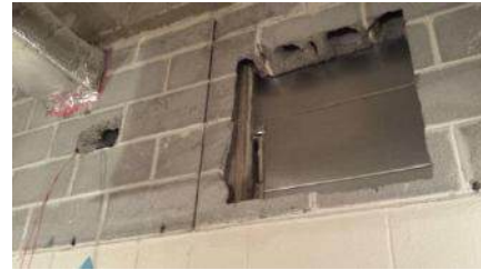
Fire wall openings
