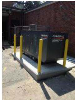
New Emergency Generator Installed
