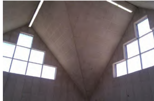
Tectum panels to be replaced
