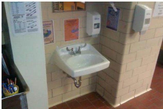
New Sinks for Wadsworth ES Kitchen
