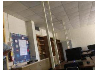
Classroom : New HVAC, Ceiling Grid to be Installed, Tile and Lighting to be Replaced
