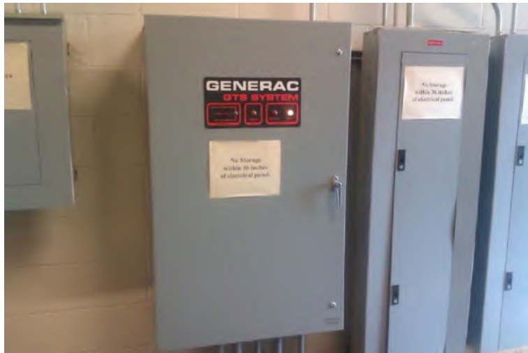
Automatic Transfer Switch to be changed out
