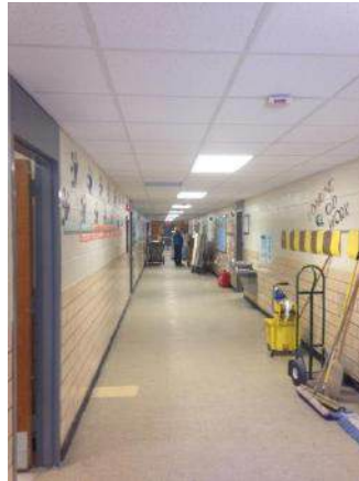
Phase 2: Main Corridor New HVAC, Ceiling Grid Installed, Tile and Lighting was Replaced
