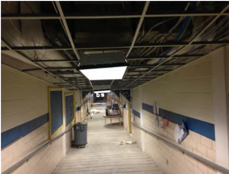
Phase 3: Main Corridor : New HVAC, Ceiling Grid to be Installed, Tile and Lighting to be Replaced
