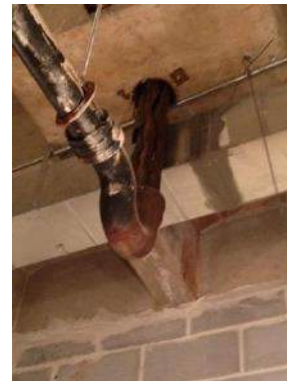
Bad piping above ceiling
