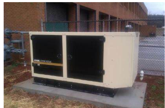
New Generator at DHST-S
