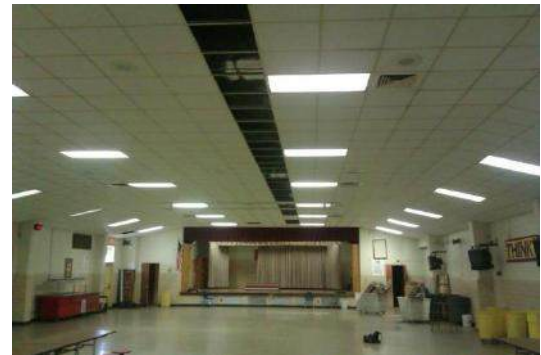
Location of power run for cafeteria lights at McNair MS
