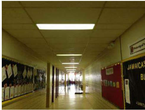
Main Corridor: New HVAC, Ceiling Grid to be Installed, and Lighting to be Replaced
