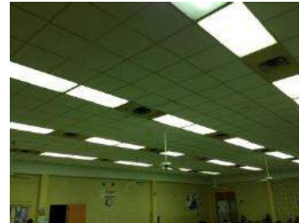
Cafeteria and Kitchen: New HVAC, Ceiling Grid to be Installed, Tile and Lighting to be Replaced
