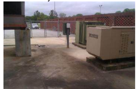
Existing Generator for Freedom MS
