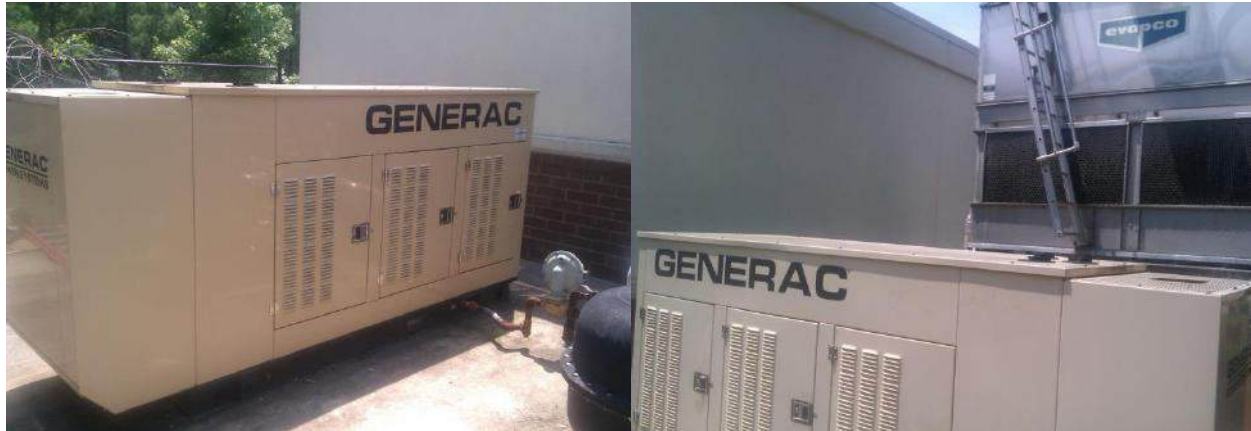
Gas Supply to Generator
