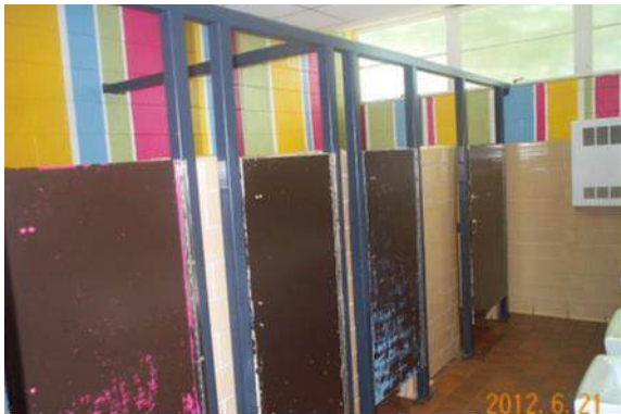
Sagamore Hills ES Existing Bathroom
