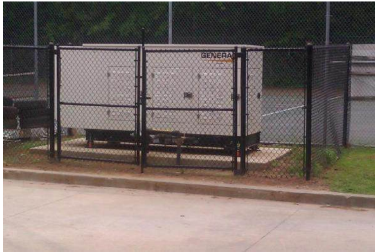
Generator serving Druid Hills HS
