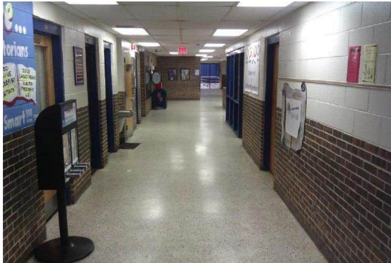
Corridor: New HVAC, Ceiling Grid to be Installed, Tile and Lighting to be Replaced
