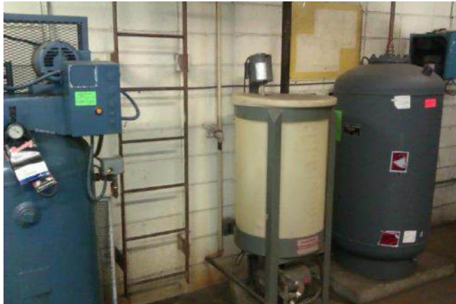
Air Compressor and water treatment equipment to be replaced
