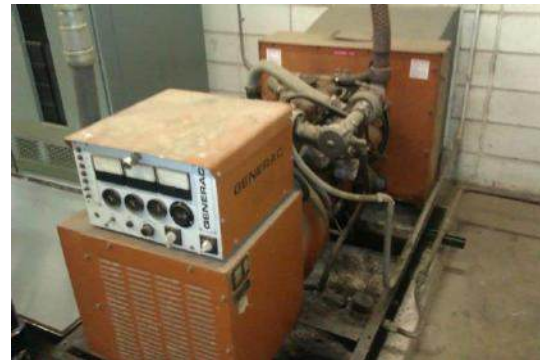
Emergency Generator to be replaced
