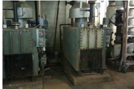
Boilers to be replacement
