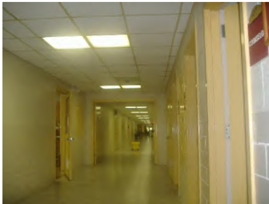
Corridor: New HVAC, Ceiling Grid to be Installed, Tile and Lighting to be Replaced
