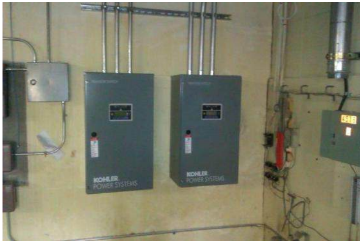
New ATS switches at Chesnut ES
