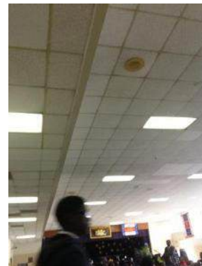
Cafeteria Ceiling Grid Covers to be Installed, Tile and Lighting to be Replaced
