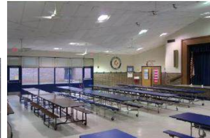
Cafeteria Center: New HVAC, Ceiling Grid to be Installed, Tile and Lighting to be Replaced
