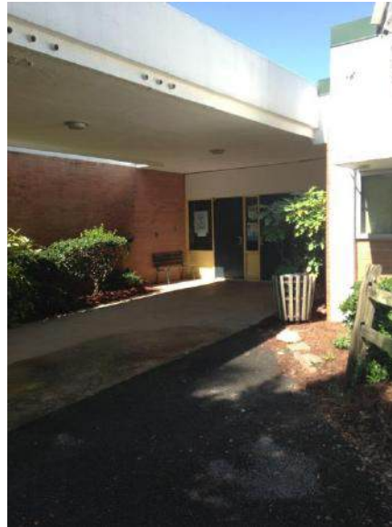
Sequoyah MS, Main Entrance Lacking ADA Access
