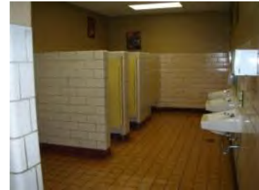
Phase 3: Bathroom : New HVAC, Ceiling Grid to be Installed, Tile and Lighting to be Replaced
