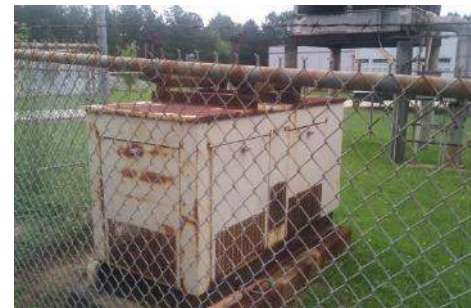
Existing Generator for Change Out
