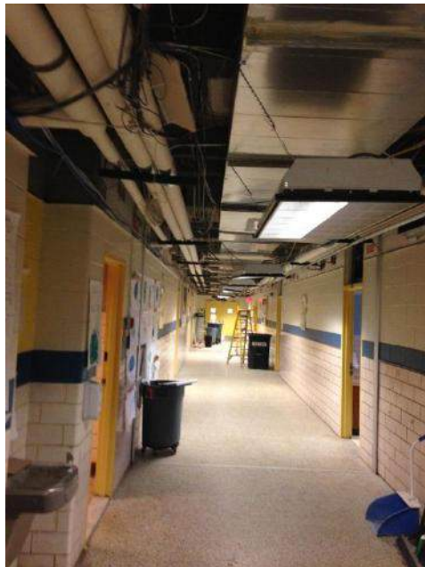
Phase 2: Main Corridor : New HVAC, Ceiling Grid to be Installed, Tile and Lighting to be Replaced
