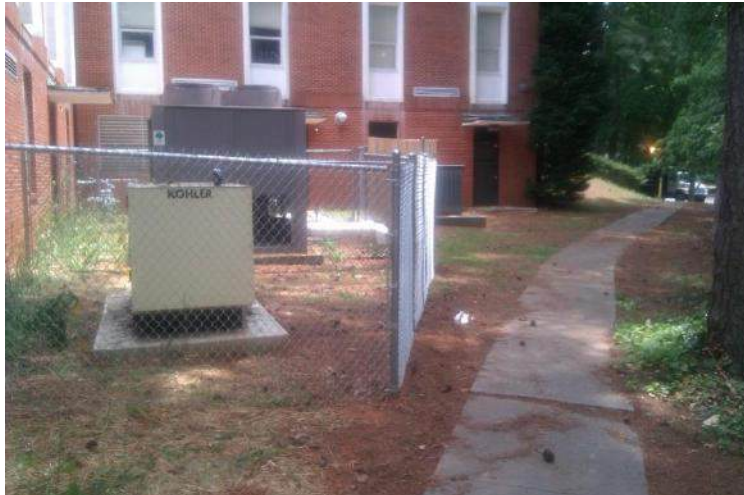
Generator and Cooling Tower Layout at Chesnut ES
