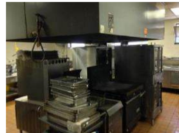
Kitchen: New HVAC, Hood, Ceiling Grid to be Installed, Tile and Lighting to be Replaced
