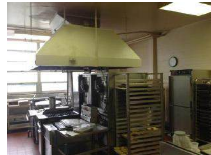
Kitchen New HVAC, Ceiling Grid to be Installed, Tile and Lighting to be Replaced
