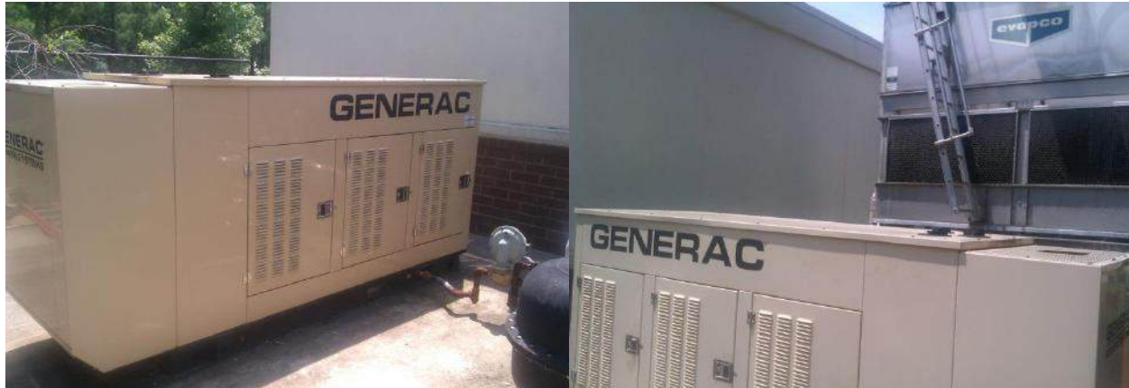
Gas Supply to Generator
