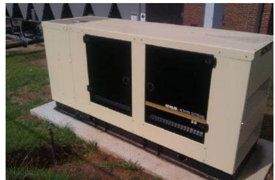
New Generator at McNair MS
