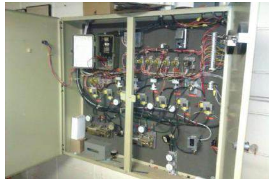
Building HVAC controls to be replaced
