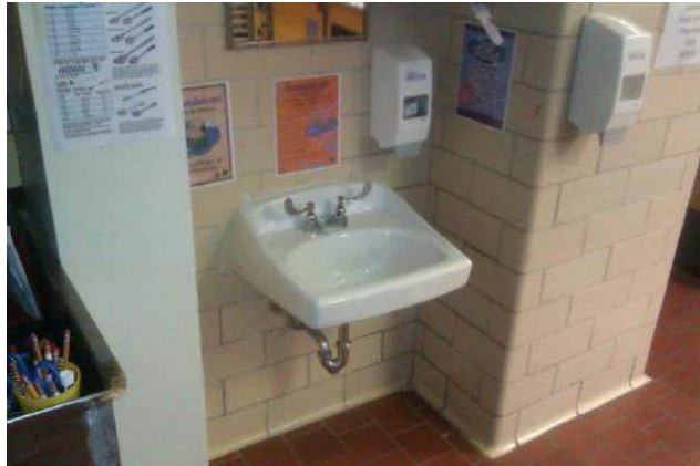
New Sinks for Wadsworth ES Kitchen
