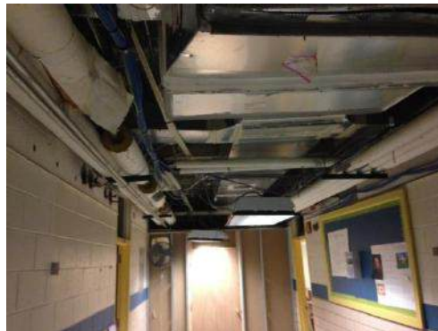
Phase 2 Construction: Main Corridor : New HVAC, Ceiling Grid to be Installed, Tile and Lighting to be Replaced
