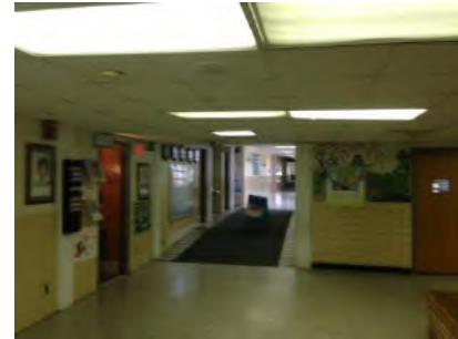
Main Corridor: New HVAC, Ceiling Grid to be Installed, Tile and Lighting to be Replaced
