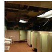
Phase 2: Bathroom : New HVAC, Ceiling Grid to be Installed, Tile and Lighting to be Replaced
