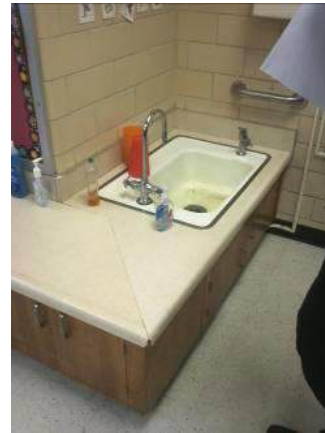
Rockbridge ES Existing Sink and Countertop
