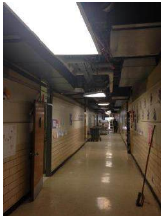
Phase 2: Main Corridor New HVAC, Ceiling Grid to be Installed, Tile and Lighting to be Replaced
