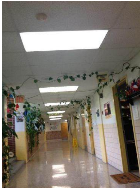
Corridor Ceiling Grid Covers to be Installed, Tile and Lighting to be Replaced
