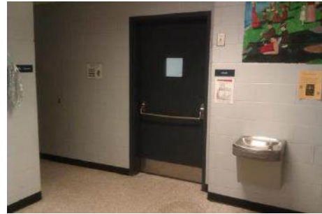
Stairwell Door for Replacement
