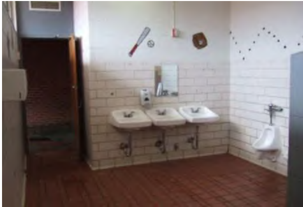
Midway ES Existing Bathroom
