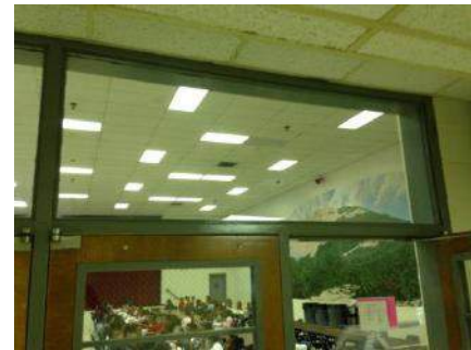
Kitchen and Cafeteria : New HVAC, Ceiling Grid to be Installed, Tile and Lighting to be Replaced
