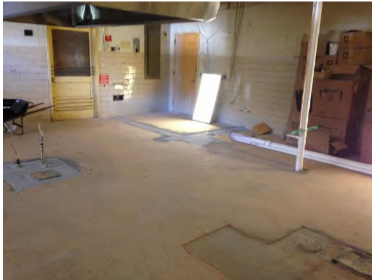
Kitchen Floor is Being Prepped for New Floor Tile, Walls and Frames are to be Painted
