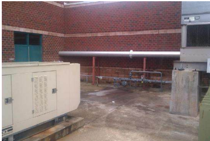
Freedom MS Generator & Gas Service
