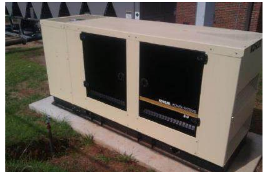
New Generator at McNair MS
