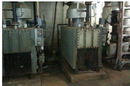
Boilers Scheduled for Replacement
