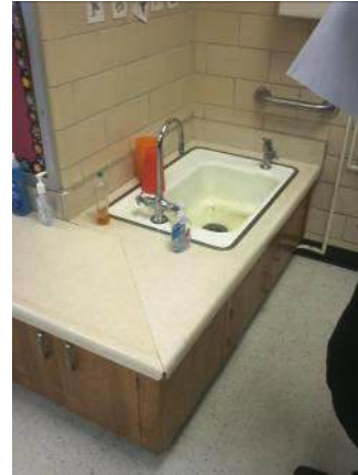
Rockbridge ES Existing Sink and Countertop
