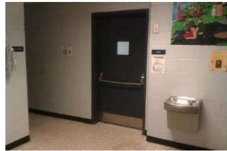
Stairwell Door for Replacement
