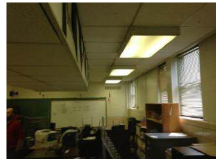
Classroom Ceiling and Lighting to be Replaced
