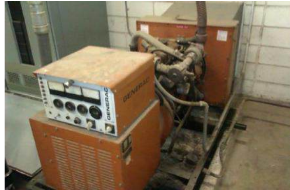
Generator Scheduled for Replacement
