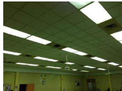
Ceiling and Lighting Fixtures
