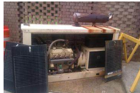
Bethune MS Generator
