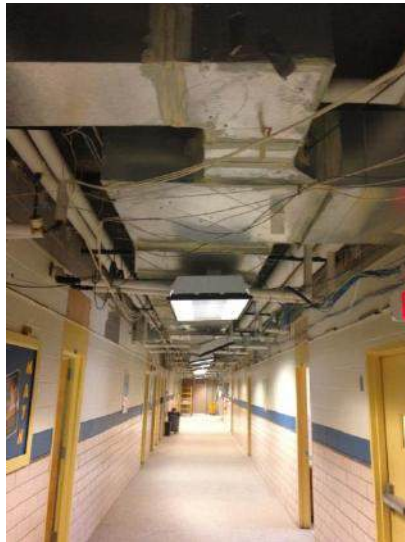
Main Corridor Lighting to be Replaced
