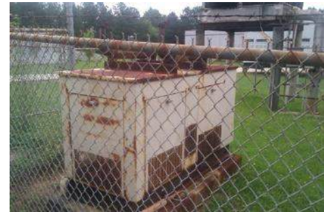
Existing Generator for Change Out
