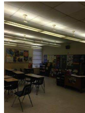
Media ceiling to be Replaced
