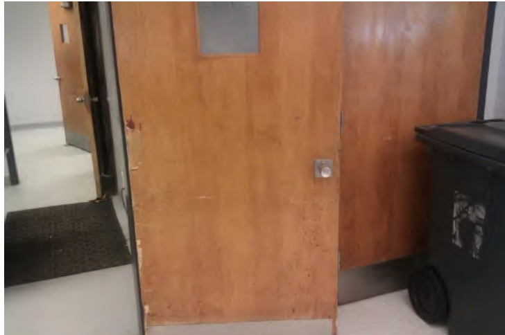
Example of Door for Replacement
