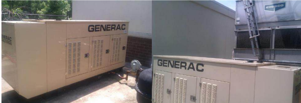
Gas Supply to Generator
