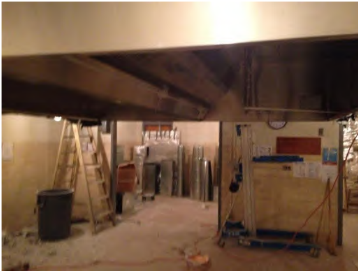
Kitchen Exhaust Hood
