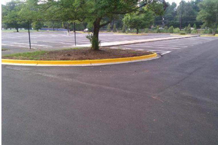
New Paint for Curb and Parking Spaces
