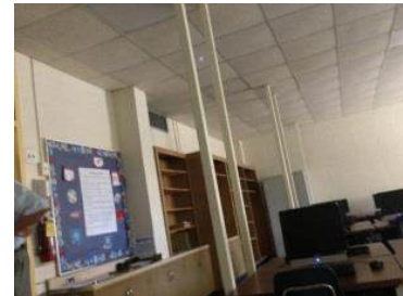
Classroom Lighting to be Replaced
