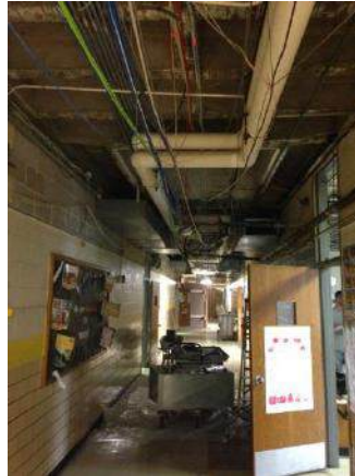
Corridor HVAC, Ceiling and Lighting to be Replaced
