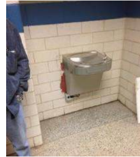
Fire Chaulking around Water Fountain and in all Above Ceiling Penetrations along the Fire Rated Walls
