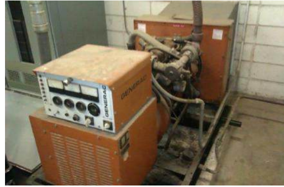
Generator Scheduled for Replacement
