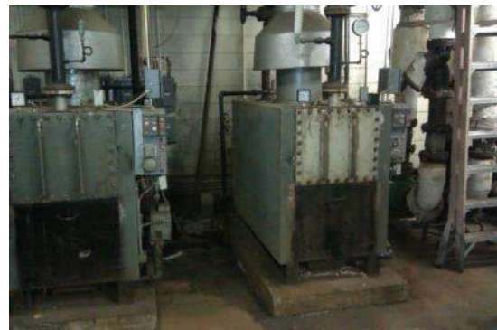
Boilers Scheduled for Replacement
