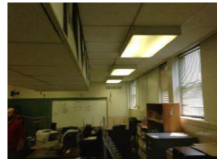
Classroom Ceiling and Lighting to be Replaced
