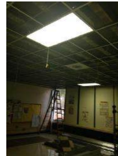
Class room HVAC, Ceiling and Lighting to be replaced
