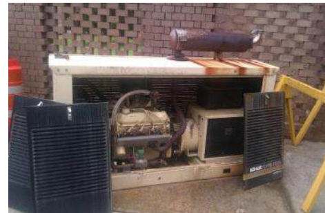
Bethune MS Generator
