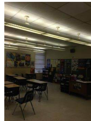
Media ceiling to be Replaced
