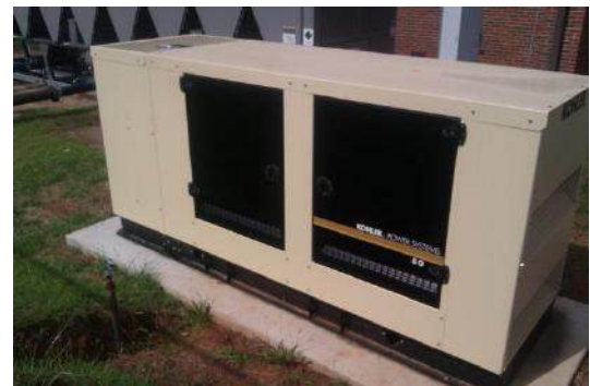
New Generator at McNair MS
