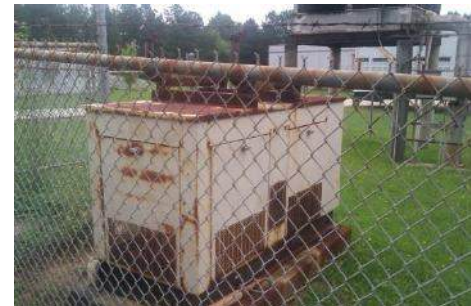
Existing Generator for Change Out
