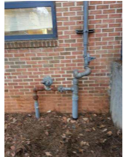
Montclair ES Gas Feed to Bldg
