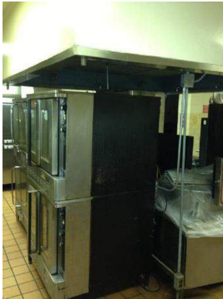
Kitchen Exhaust Hood
