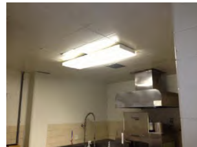
Kitchen Exhaust Hood
