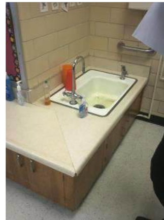
Rockbridge ES Existing Sink and Countertop
