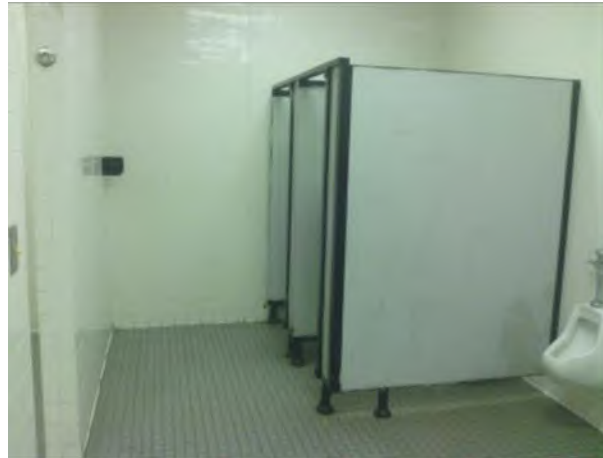
Salem MS Existing Gym Bathroom
