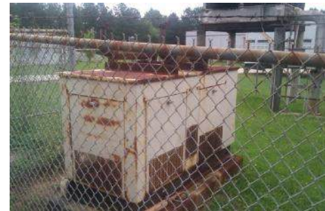
Existing Generator for Change Out
