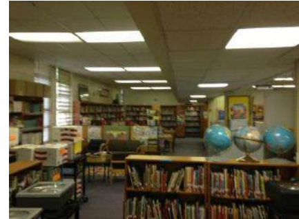
Media Center Lighting to be Replaced
