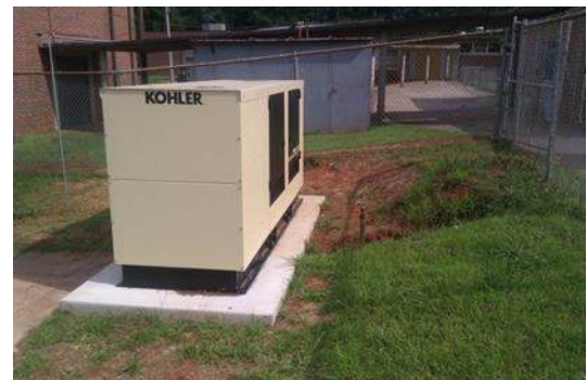
New Generator at McNair MS
