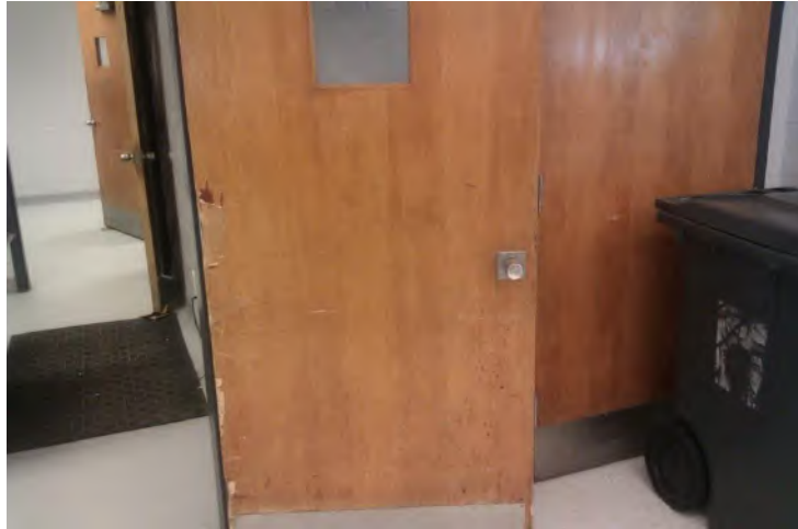
Example of Door for Replacement
