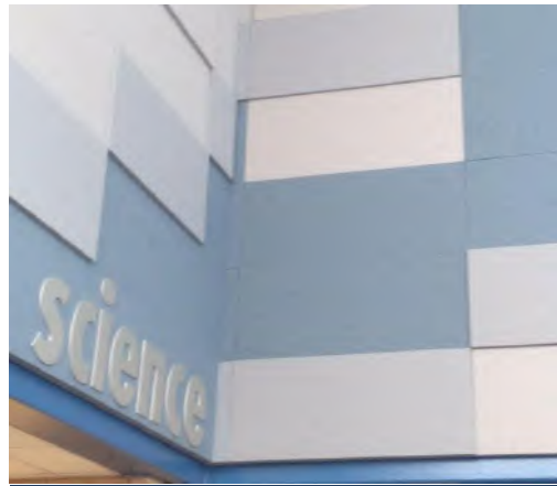
New Acoustical Panels
