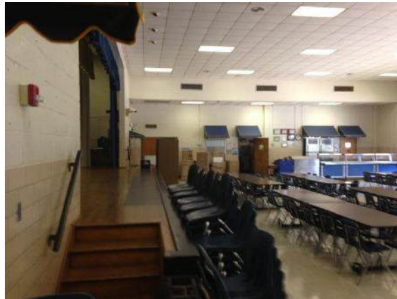
Cafeteria Lighting to be Replaced
