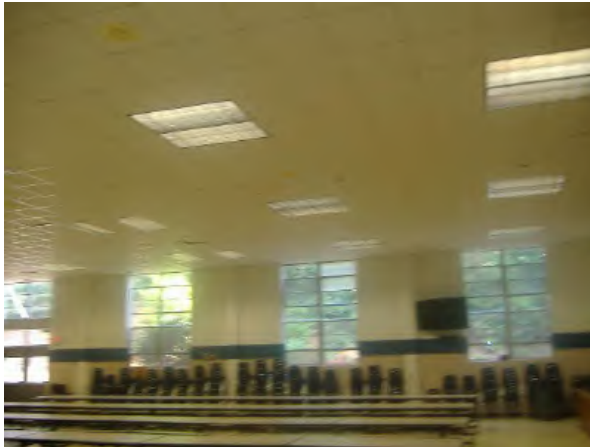
Ceiling Lighting and HVAC to be Replaced
