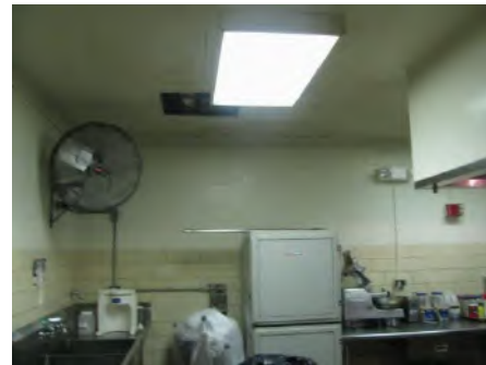
Kitchen Hood and Lighting
