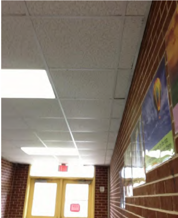
Hall Ceiling and Lighting to be Replaced
