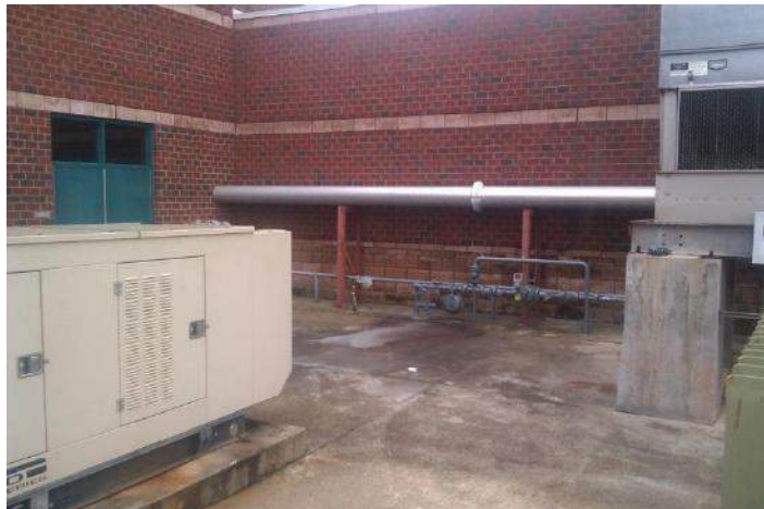
Freedom MS Generator & Gas Service
