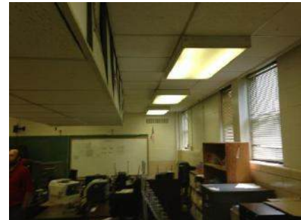
Classroom Ceiling and Lighting to be Replaced
