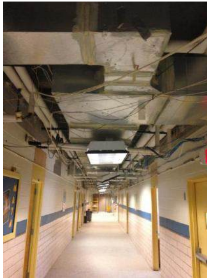
Main Corridor Lighting to be Replaced
