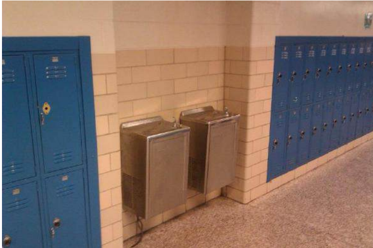
Water Coolers to be Replaced
