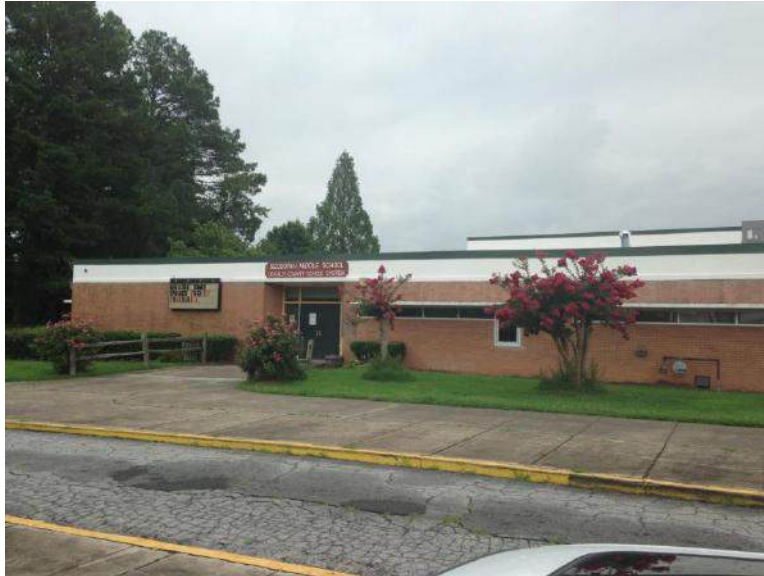
ADA Access from Parking Lot to the Front of the School Building is Needed
