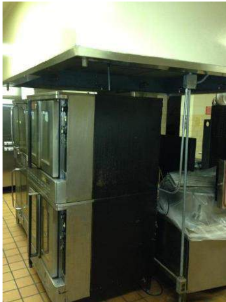
Kitchen Exhaust Hood
