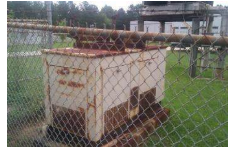
Existing Generator for Change Out
