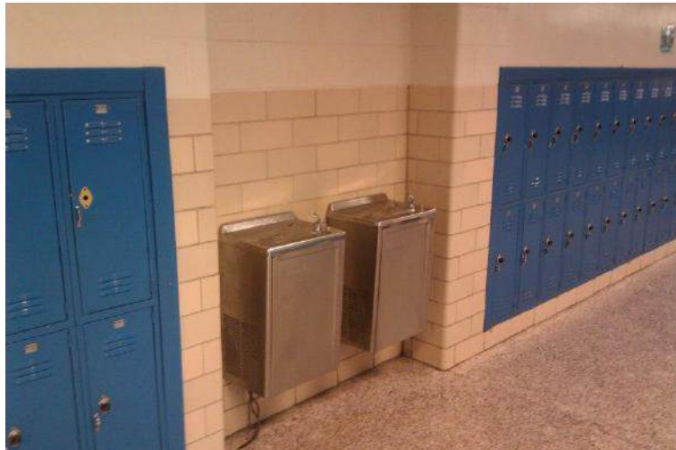
Water Coolers to be changed out
