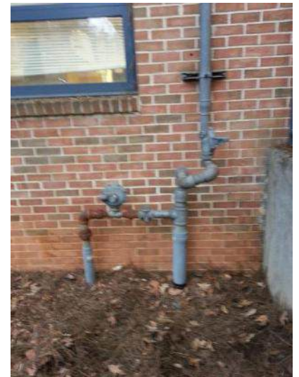
Montclair ES Gas Feed to Bldg
