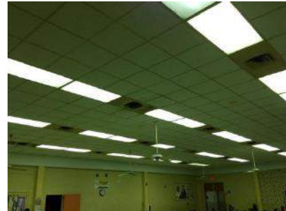
Ceiling and Lighting Fixtures
