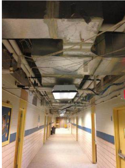
Main Corridor Lighting to be Replaced
