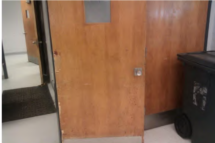
Example of Door for Replacement
