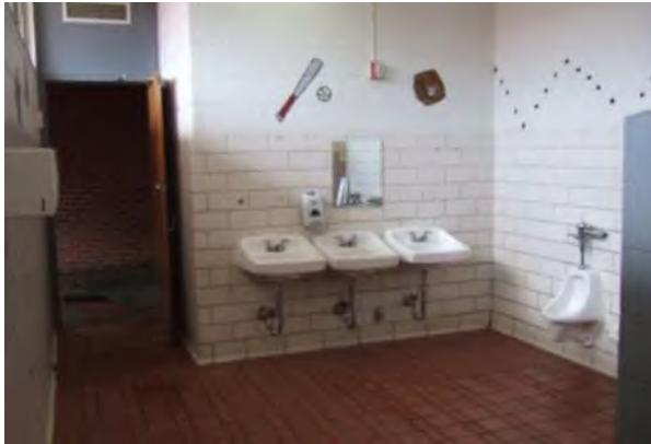
Midway ES Existing Bathroom
