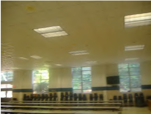
Ceiling Lighting and HVAC to be Replaced
