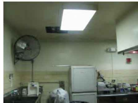
Kitchen Hood and Lighting
