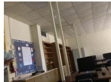
Classroom Lighting to be Replaced
