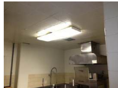
Kitchen Exhaust Hood
