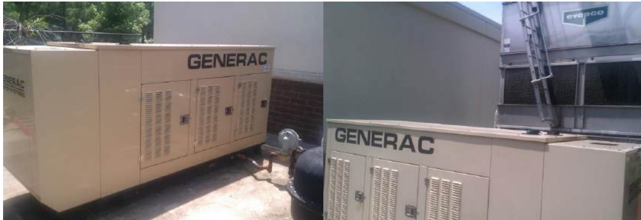
Gas feed to generator
