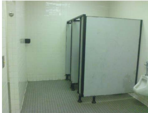
Salem MS Existing Gym Bathroom
