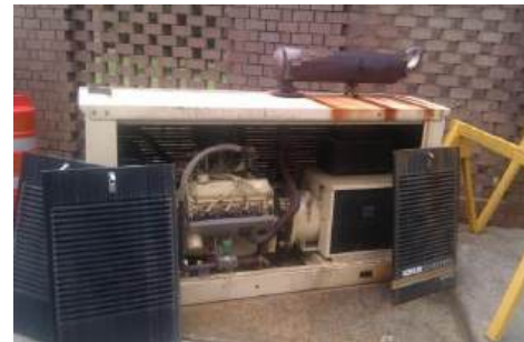
Bethune MS Generator
