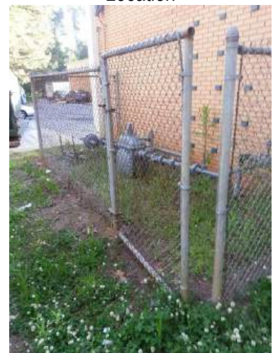
Canby Lane ES Gas Meter Location
