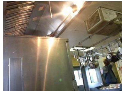
Kitchen Hood, Ceiling Lighting and HVAC to be Replaced in the Kitchen
