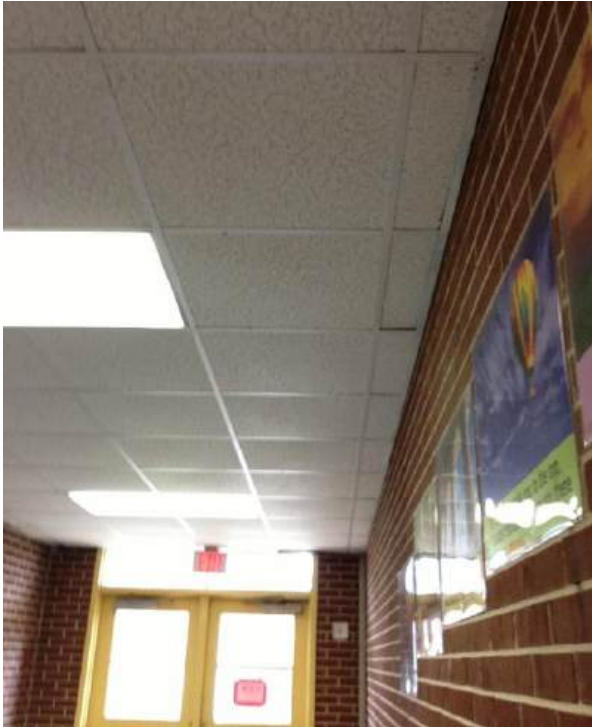
Hall Ceiling and Lighting to be Replaced
