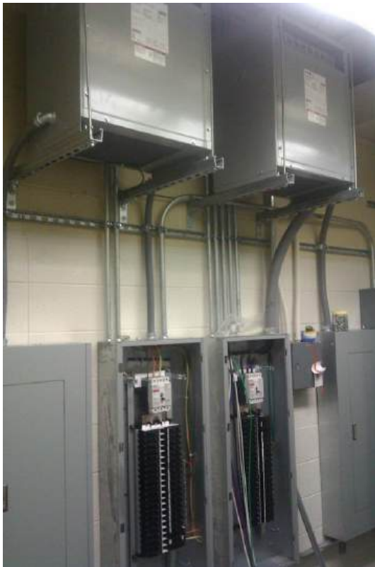
New Panels and Transformers at DHST-S
