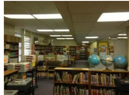
Media Center Lighting to be Replaced
