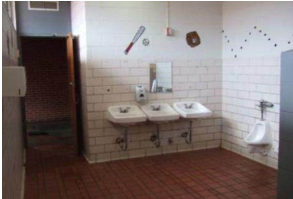
Midway ES Existing Bathroom
