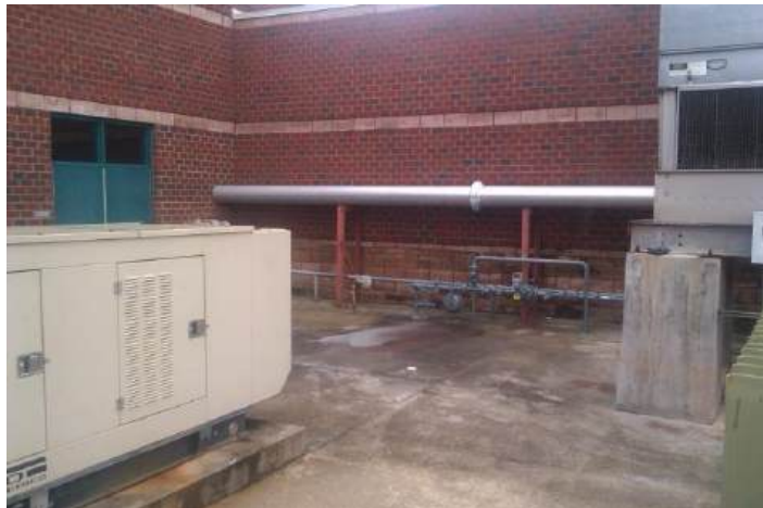
Freedom MS Generator & Gas Service
