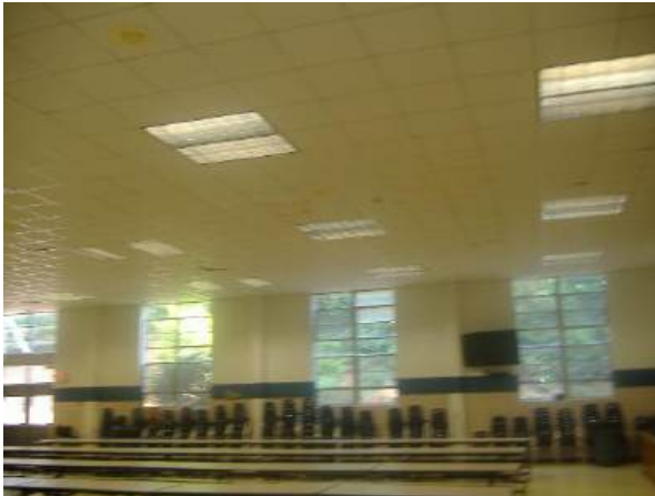
Ceiling Lighting and HVAC to be Replaced
