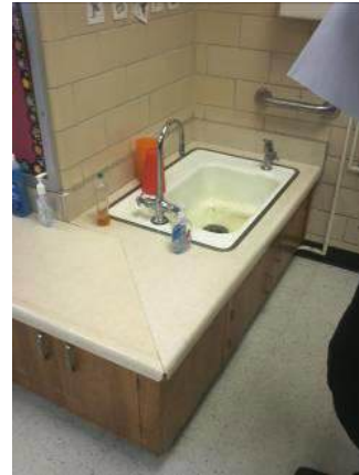
Rockbridge ES Existing Sink and Countertop
