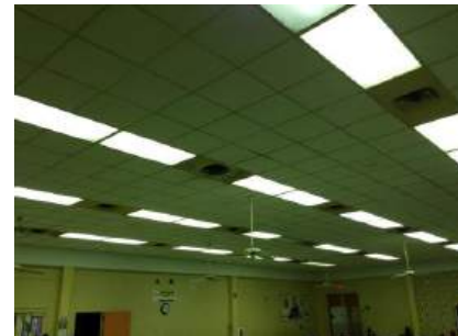
Ceiling and Lighting Fixtures
