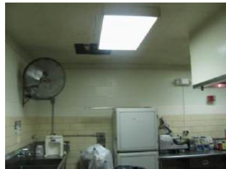
Kitchen Hood and Lighting
