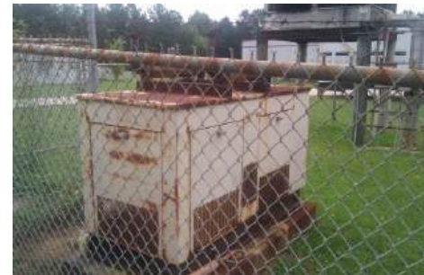
Existing Generator for Change Out
