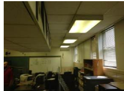
Classroom Ceiling and Lighting to be Replaced
