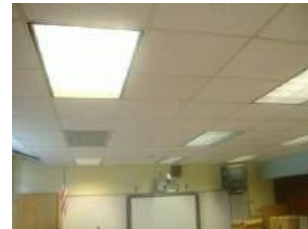
Classroom Lighting to be Replaced
