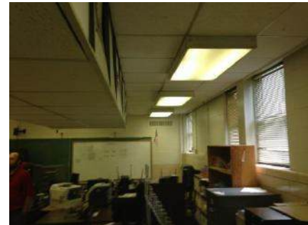
Classroom Ceiling and Lighting to be Replaced
