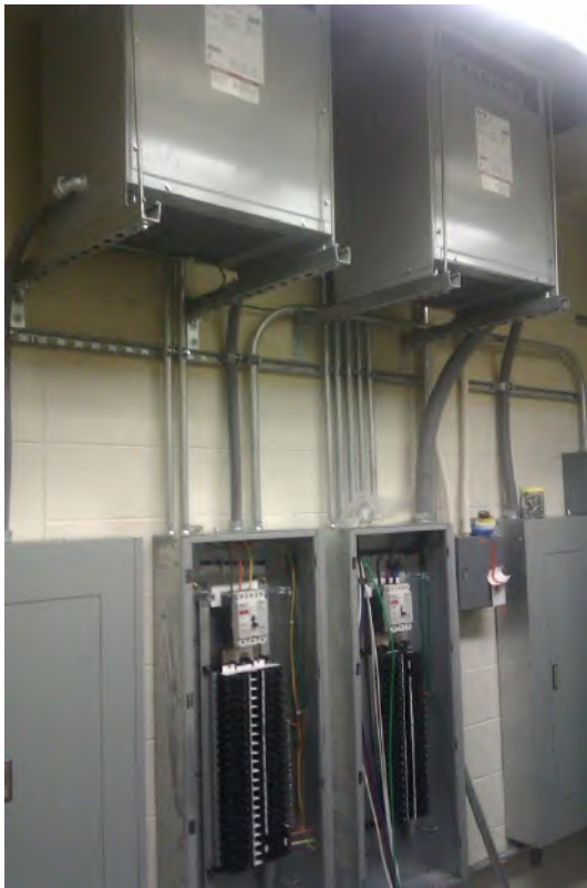
New Panels and Transformers at DHST-S
