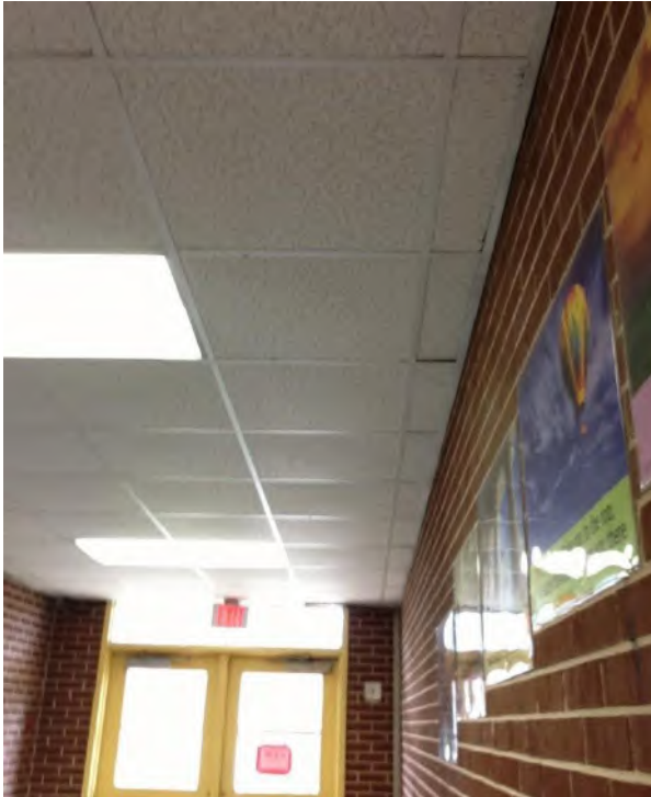
Hall Ceiling and Lighting to be Replaced
