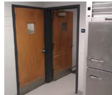
Kitchen Doors for Replacement
