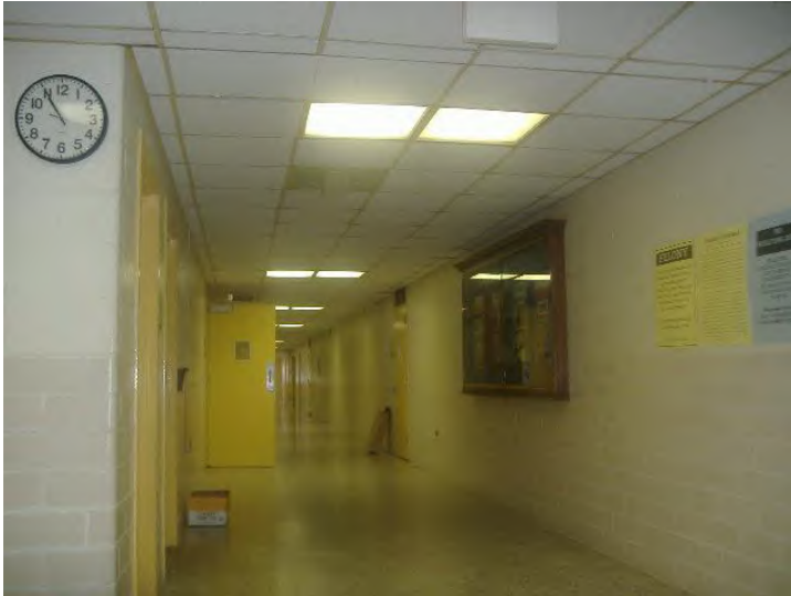
Main Corridor Lighting to be Replaced
