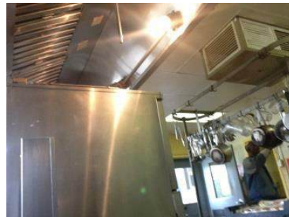
Kitchen Hood, Ceiling Lighting and HVAC to be Replaced in the Kitchen
