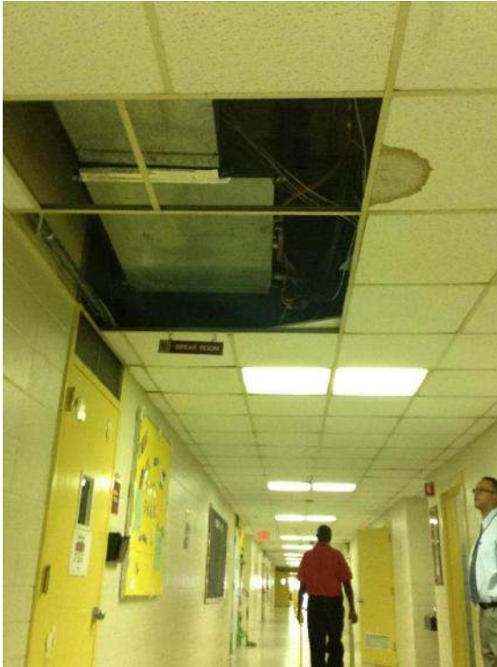
Hall Lighting to be Replaced
