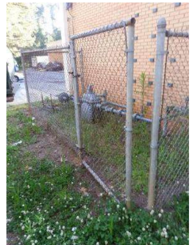
Canby Lane ES Gas Meter Location
