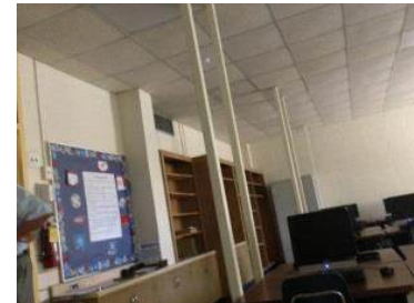
Classroom Lighting to be Replaced
