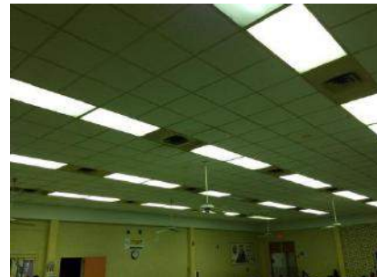
Ceiling and Lighting Fixtures
