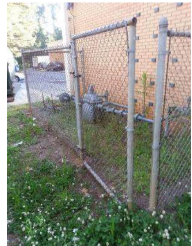
Canby Lane ES gas meter location
