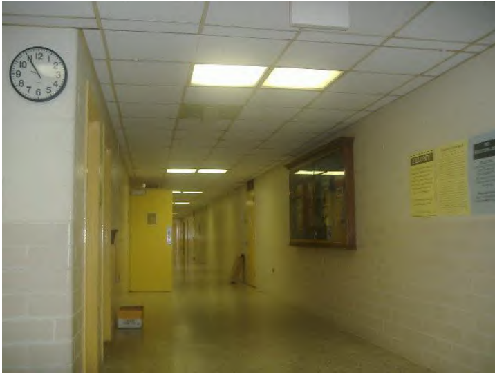
Main corridor lighting to be replaced
