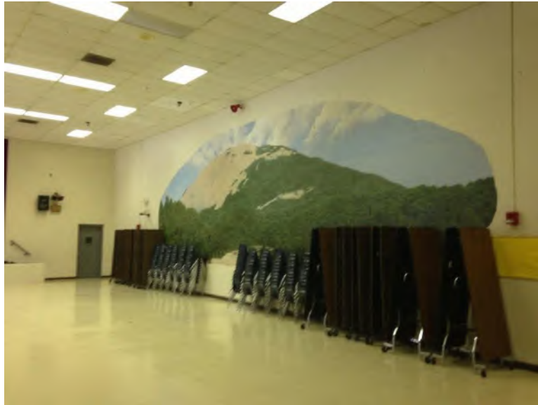
Cafeteria ceiling and lighting to be replaced
