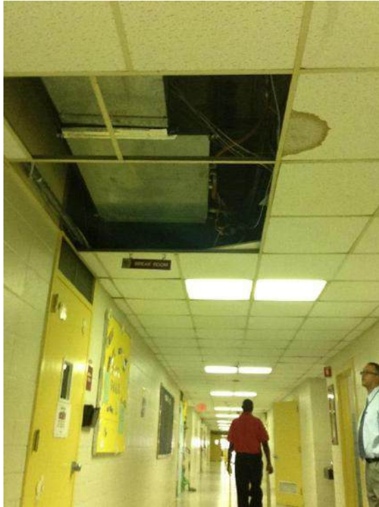
Hall Lighting to be replaced
