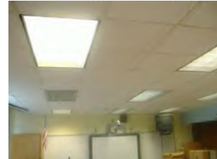
Classroom lighting to be replaced
