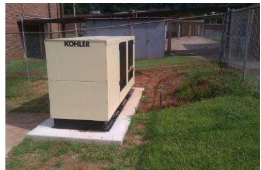
New Generator at McNair MS
