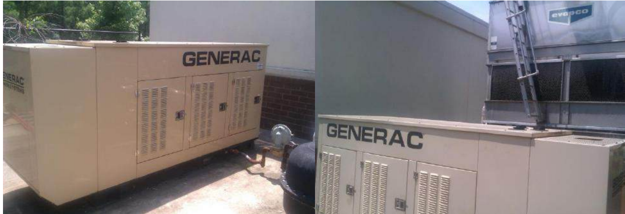
Gas feed to generator
