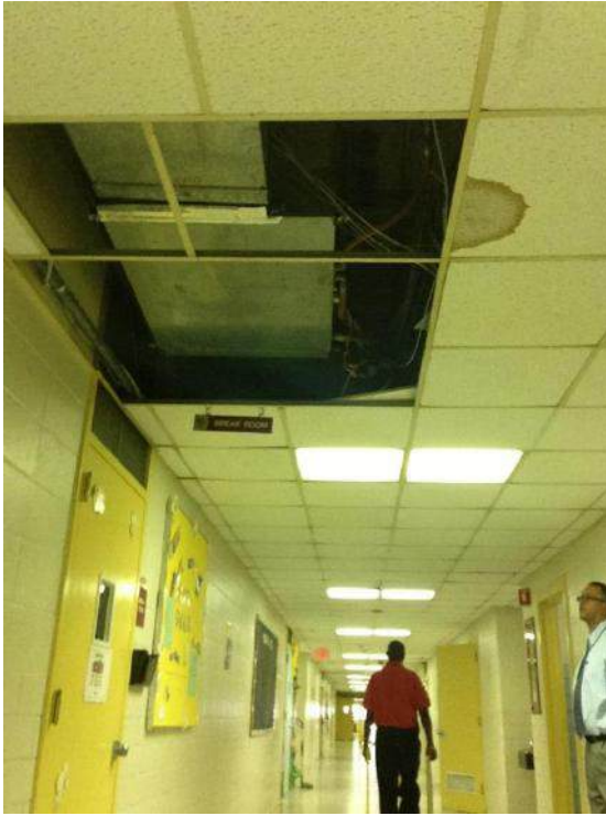
Hall Lighting to be replaced
