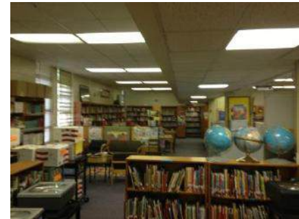
Media Center lighting to be Replaced
