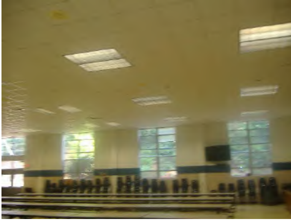
Ceiling Lighting and HVAC to be Replaced
