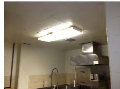
Kitchen Exhaust Hood
