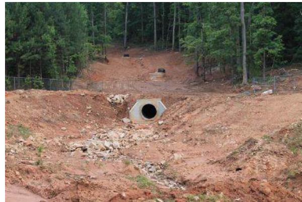
Storm Water Line to Detention Pond
