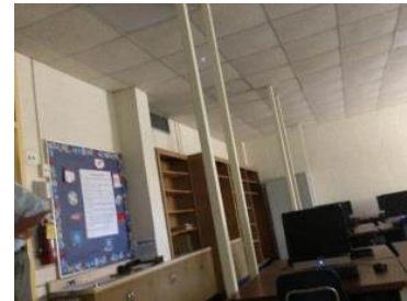
Classroom Lighting to be Replaced
