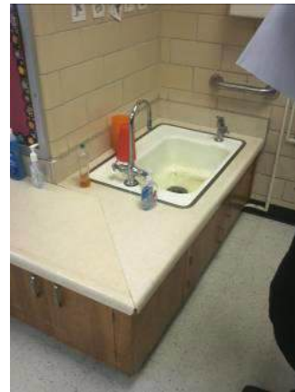
Rockbridge ES Existing Sink and Countertop
