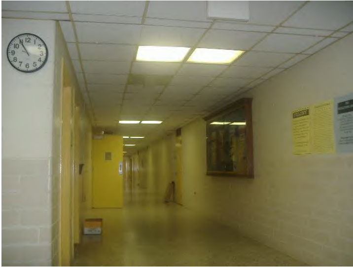
Main corridor lighting to be replaced
