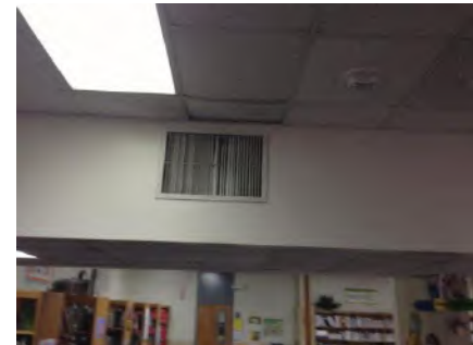
Classroom Lighting to be Replaced
