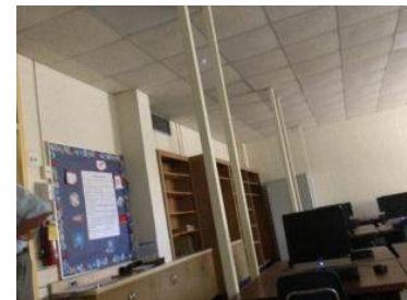
Classroom Lighting to be Replaced
