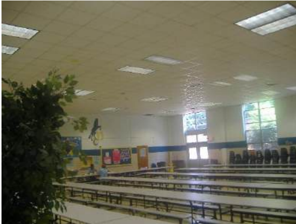
Cafeteria Lighting to be Replaced
