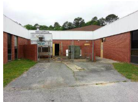
Cedar Grove ES mechanical yard
