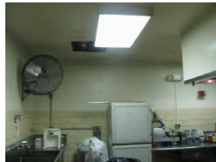
Kitchen Hood and Lighting
