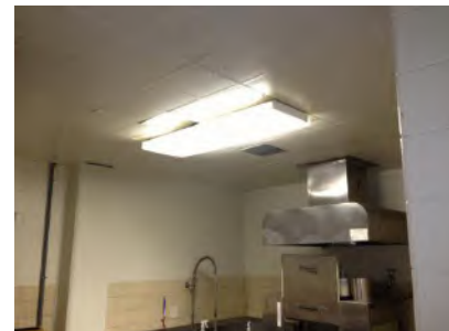
Kitchen Exhaust Hood
