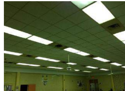
Ceiling and Lighting Fixtures
