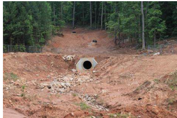
Storm Water Line to Detention Pond
