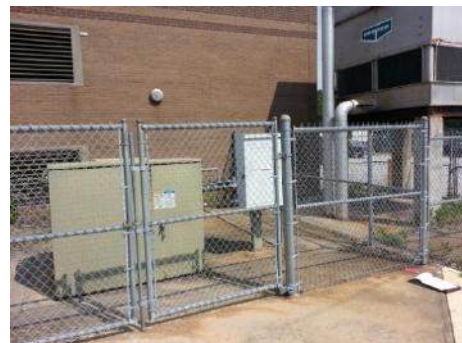
Shadow Rock ES possible generator location
