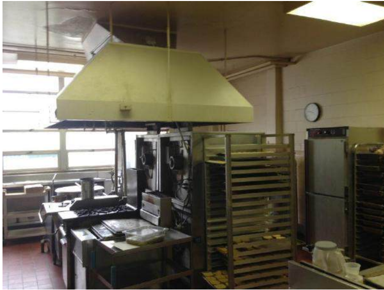
Kitchen Exhaust Hood
