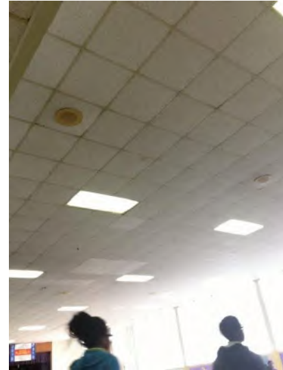
Cafeteria Lighting to be Replaced
