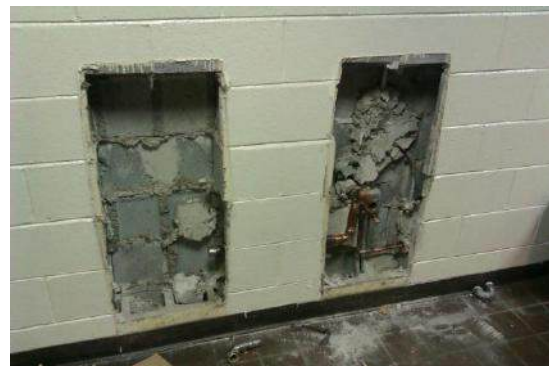
New water cooler location
