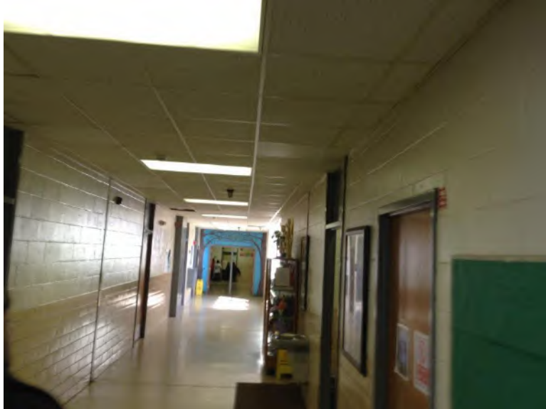
Main Corridor Lighting to be Replaced
