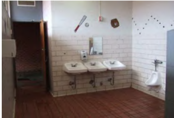
Midway ES Existing Bathroom
