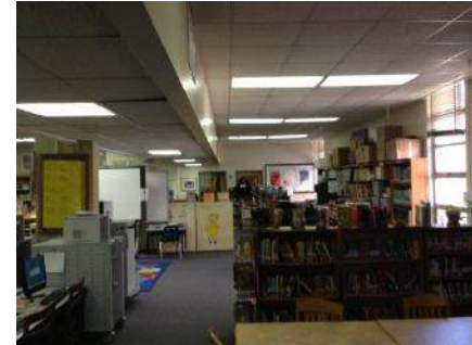
Media Center lighting to be Replaced
