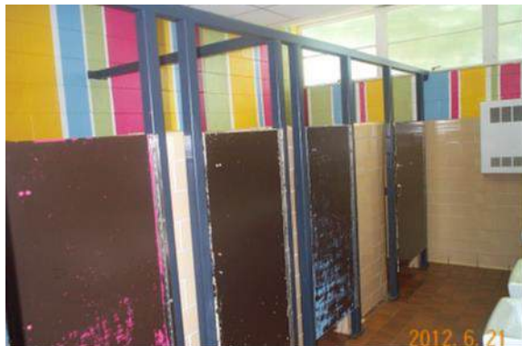
Sagamore Hills ES Existing Bathroom
