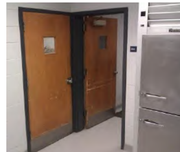
Kitchen doors for replacement
