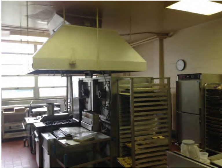
Kitchen Exhaust Hood
