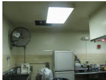
Kitchen Hood and Lighting
