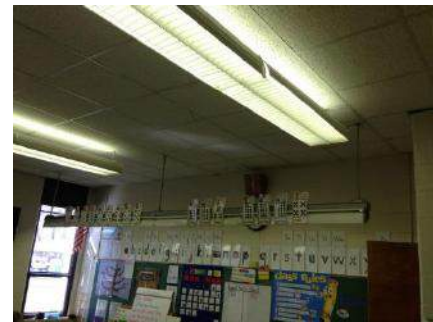
Classroom Lighting to be Replaced
