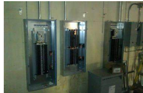
New Breaker Panels for Chesnut ES
