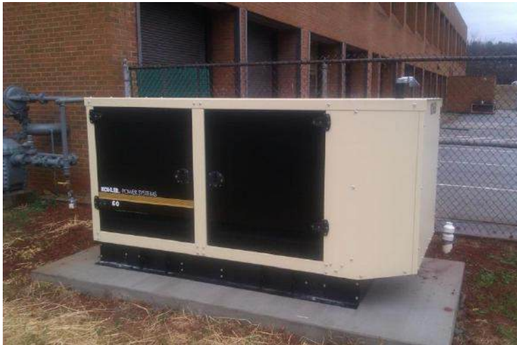
New Generator at DHST-S
