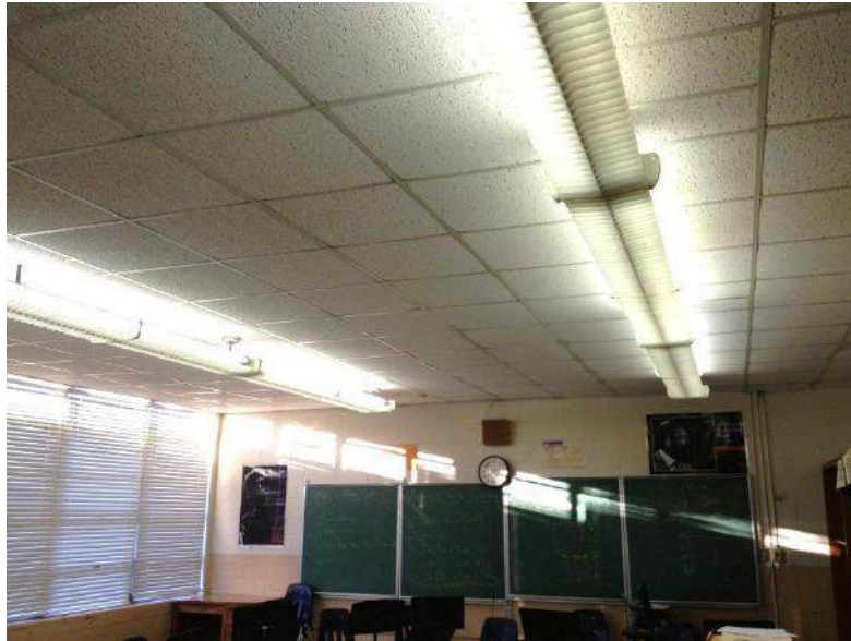
Classroom Lighting to be Replaced
