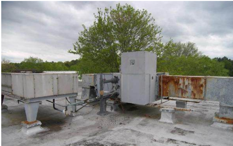
Existing HVAC above Media Center to be Replaced
