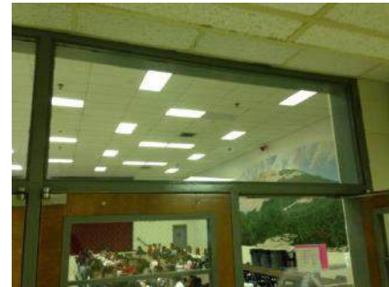
Cafeteria Lighting to be Replaced
