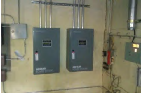
ATS switches for Chesnut ES
