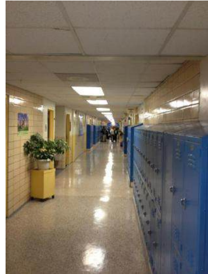
Hall Lighting to be Replaced
