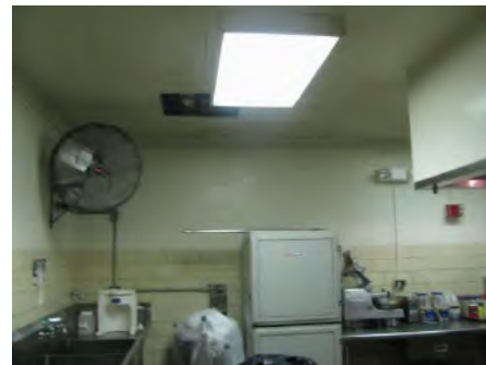
Kitchen Hood and Lighting
