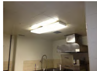
Kitchen Exhaust Hood
