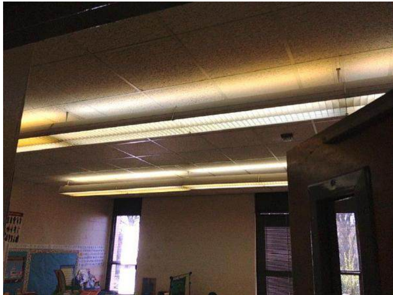
Classroom Lighting to be Replaced
