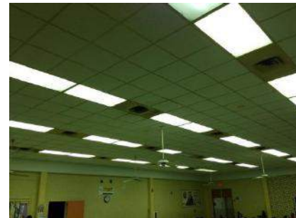
Ceiling and Lighting Fixtures
