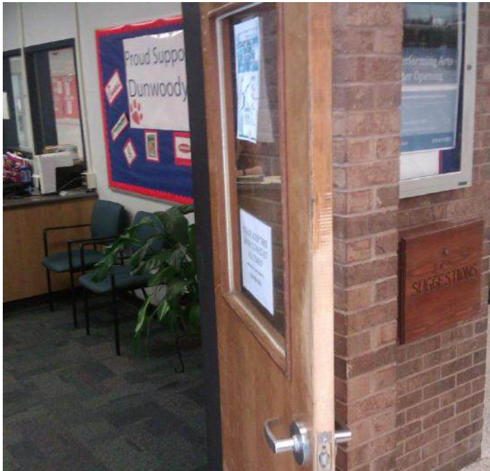
Shaved Main Office Door
