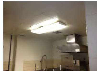
Kitchen Exhaust Hood
