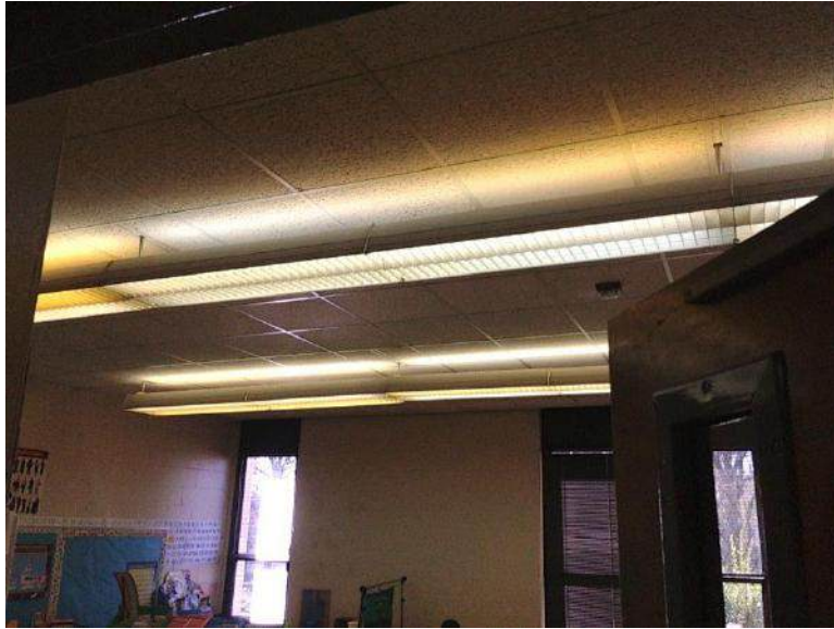
Classroom Lighting to be Replaced
