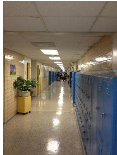
Hall Lighting to be Replaced
