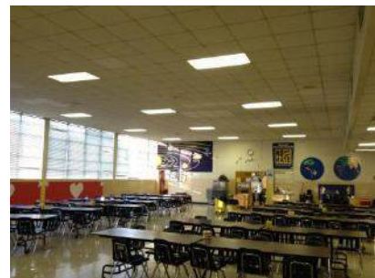
Cafeteria Lighting to be Replaced
