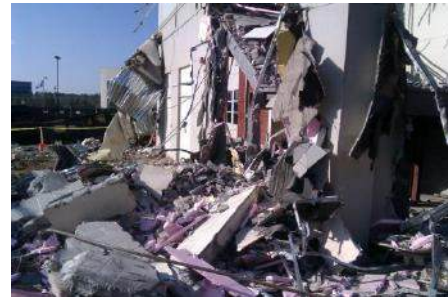
Debris from Stairwell Demolition
