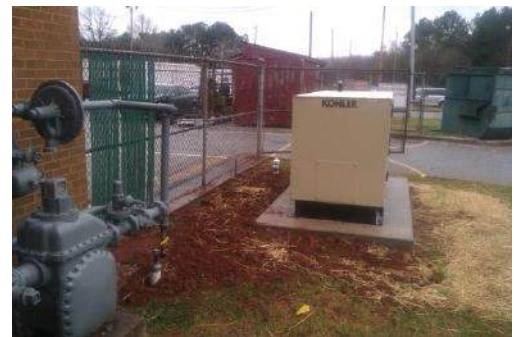
Gas to Generator
