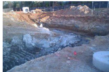
Rock Path of Storm Piping
