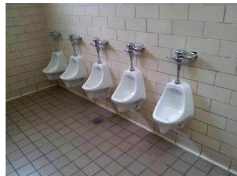
Boys' Restroom after Installation
