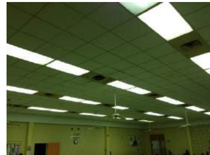
Ceiling and Lighting Fixtures
