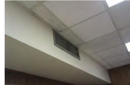
Ceiling Heating/Cooling Register
