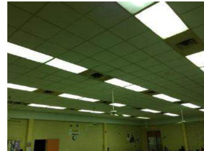
Ceiling and Lighting Fixtures
