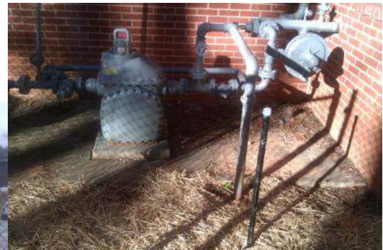
Chesnut ES -- Gas Ready for Connection
