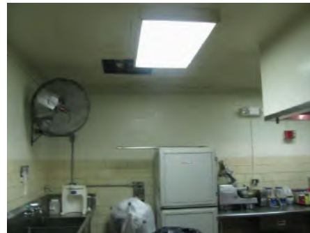
Kitchen Hood and Lighting
