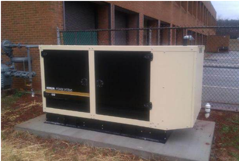
DeKalb High School of Technology - South New Generator
