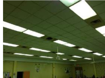
Ceiling and Lighting Fixtures
