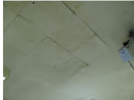
Kitchen Tiles to be Replaced
