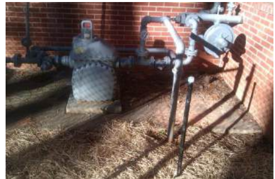
Chesnut ES -- Gas Ready for Connection
