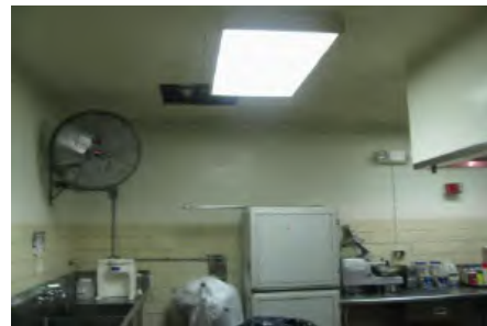
Kitchen Hood and Lighting
