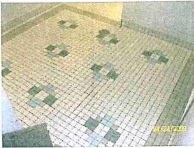
(Tile on Bathroom floor )
