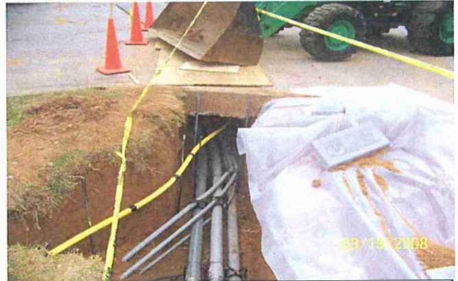
Jolly ES New Electrical Service
