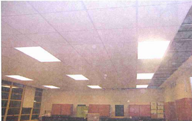
Avondale HS Ceiling Grid & Lighting
