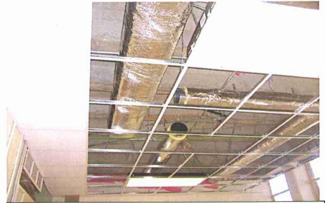
Avondale HS Supply Ducts
