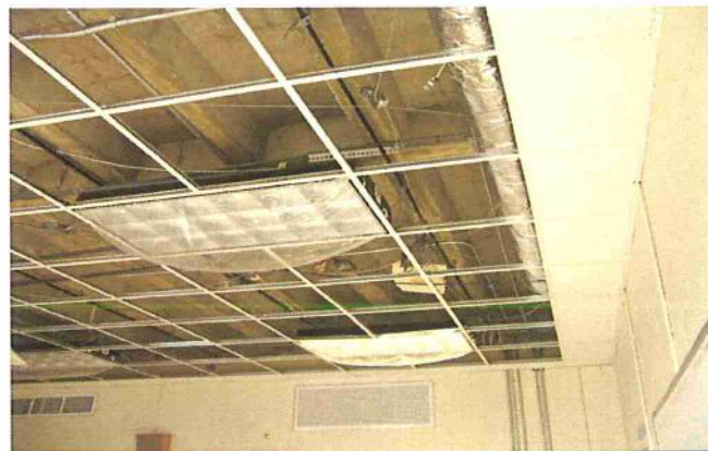
Avondale HS Ceiling Grid & Air Duct
